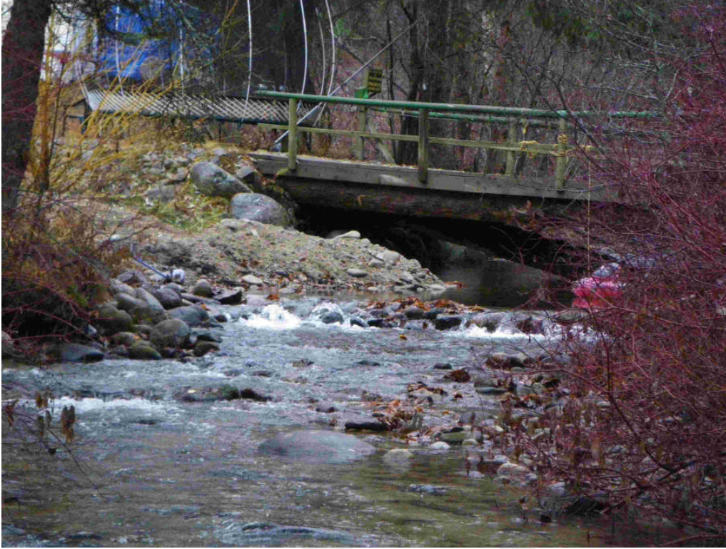
Photo 11. Private bridge with collapsed stringer visible under bridge deck compromising crossing capacity. Note gravel pushed into the creek from private property.
