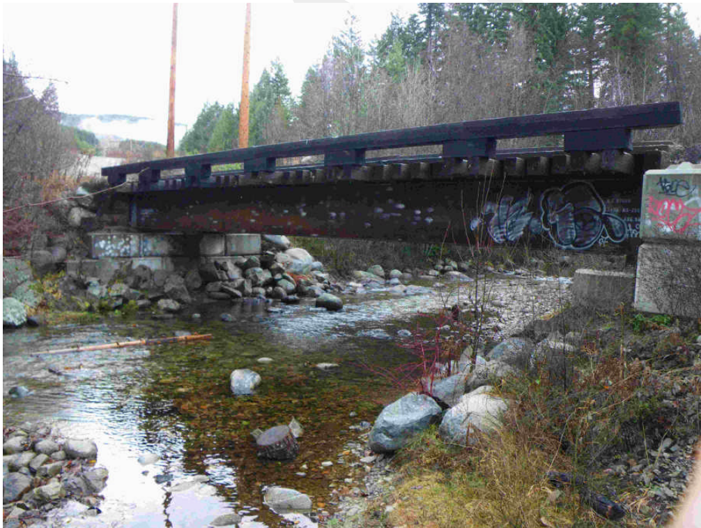
Photo 10. Forestry road crossing of Trepanier Creek 1.4 km upstream of DOP intake. Steel span bridge with lock block abutments.
