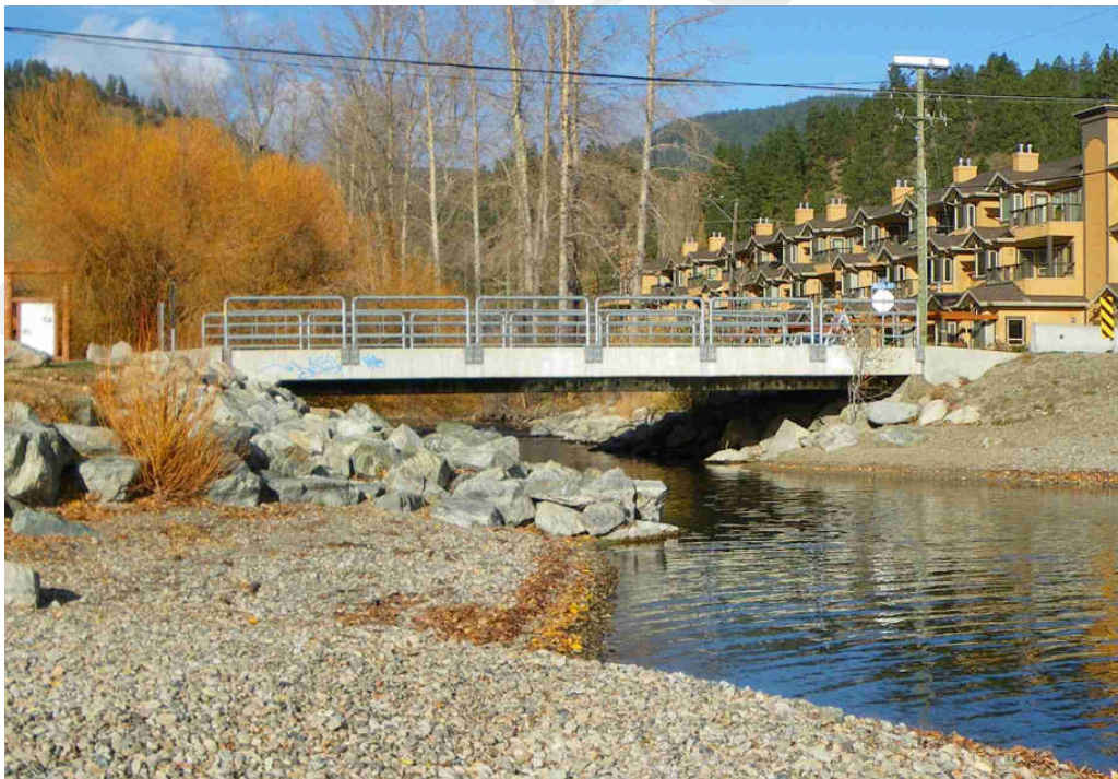
Photo 12. Beach Avenue bridge on the shoreline of Okanagan Lake. Limited bridge capacity could be reduced by channel aggradation on the fan
