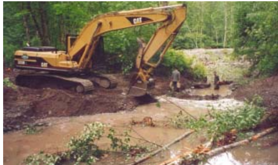
Figure 2. Moving an isolation barrier between new work (foreground) and existing habitat; and changing from earthworks to sandbags
