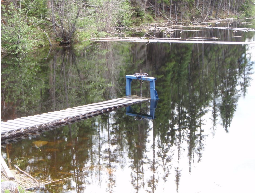
Figure 34. View from dam on Nicklen Lake to screw gate which controls the water release valve.
