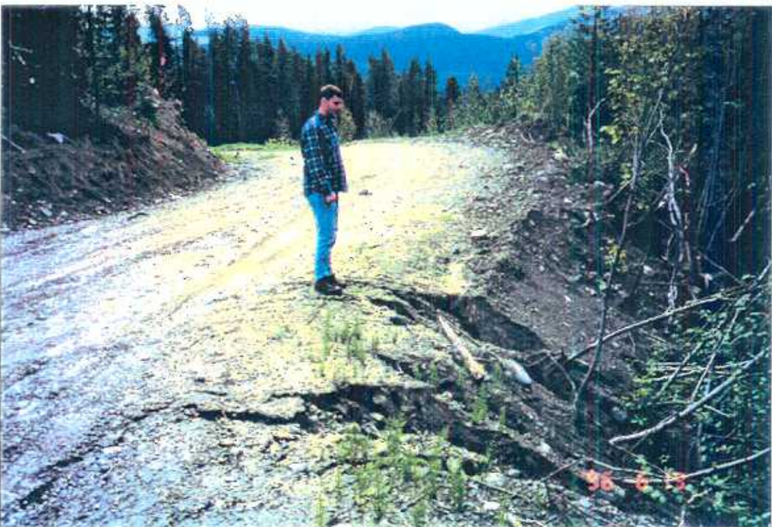
PHOTO 34. Road fill erosion in the Upper Trout Creek sub-basin. (June 1996 - ID# 1-6)
