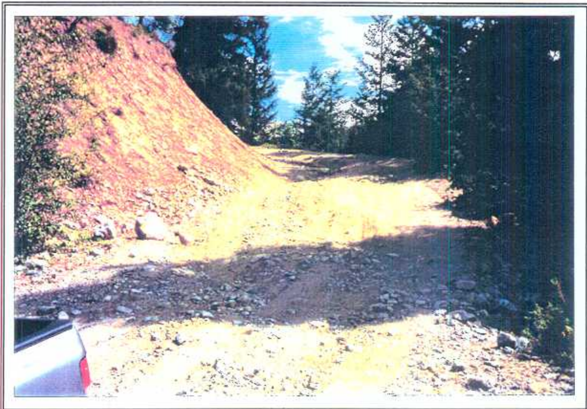
PHOTO 4. Road surface erosion directly above Darke Lake in the Darke Lake Park. (June 1996 - ID# 6-5)
