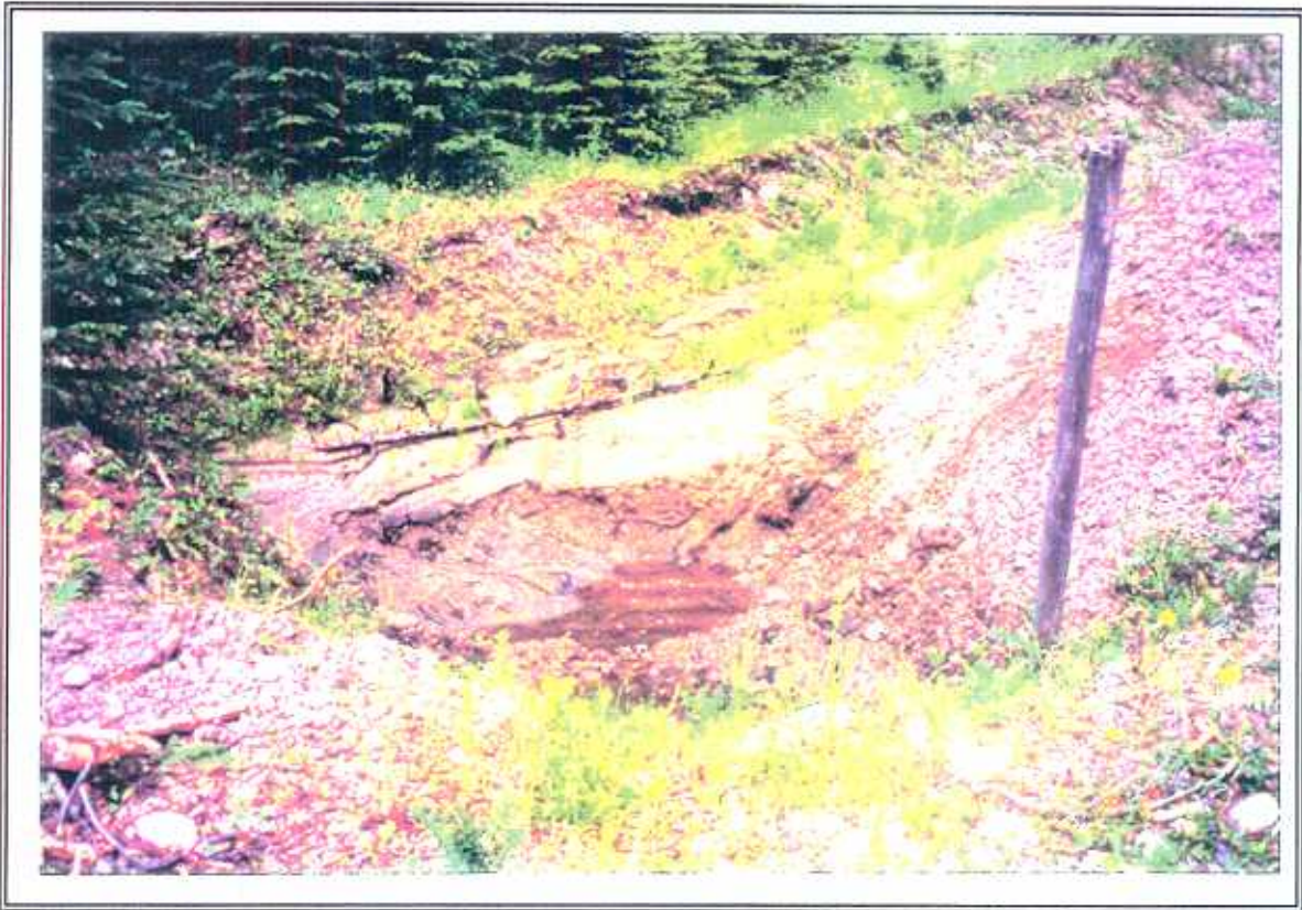
PHOTO 18. Sediment deposition in a ditch adjacent to Glen Lake Main. (June 1996 - ID# 4-7)
