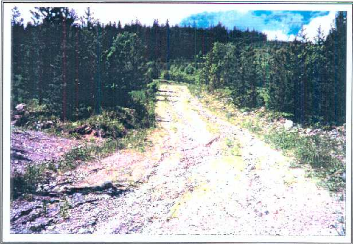
PHOTO 19. Road surface erosion on the access road to the powerline in the Camp Creek sub-basin. (June 1996 - ID# 4-13)
