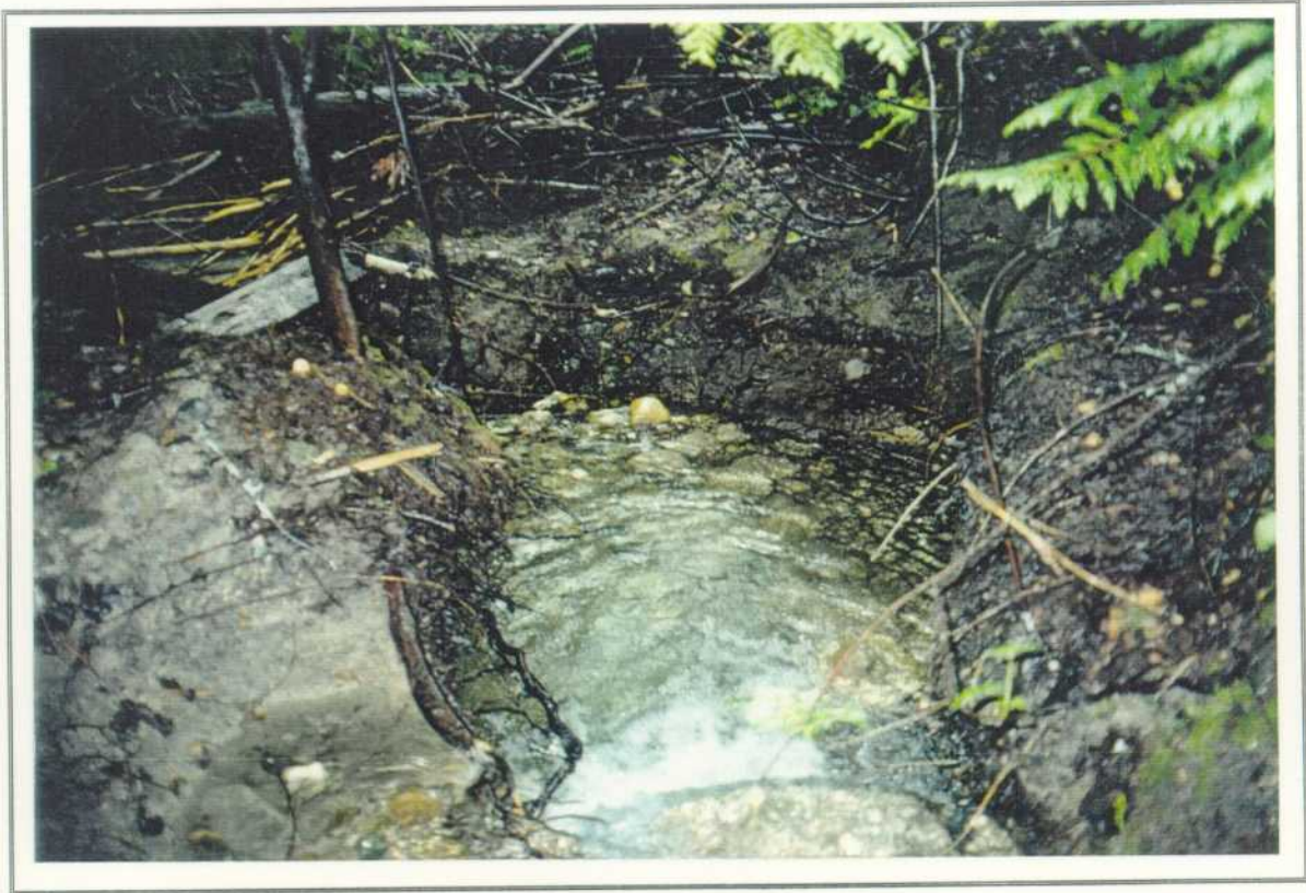
PHOTO 7. Evidence of channel bank erosion and scour below POI at lower road crossing location.
