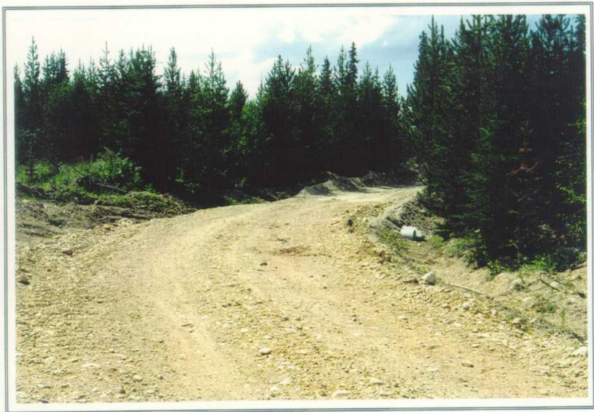
PHOTO 2. New road on the plateau section of the watershed. Coarse surfaced and well drained.
