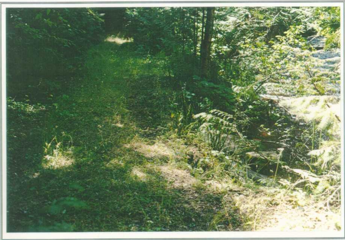
PHOTO 27. Minor channel bank erosion and road fill input to the channel on old trail upstream of Headgates reservoir.
