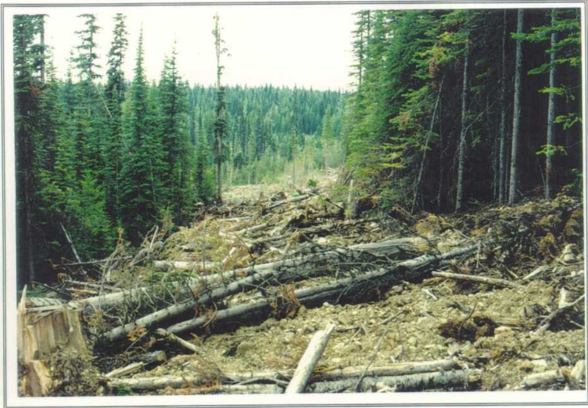
PHOTO 1. Temporary access structure (road) from Aberdeen FSR to recent cutblock upslope of canyon section.
