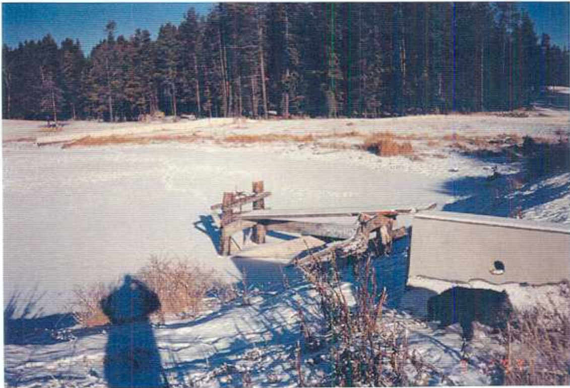
Plate 8: (Site 4) Dam on Leighton Lake to control water flow into Tunkwa Creek (December 9, 1997)
