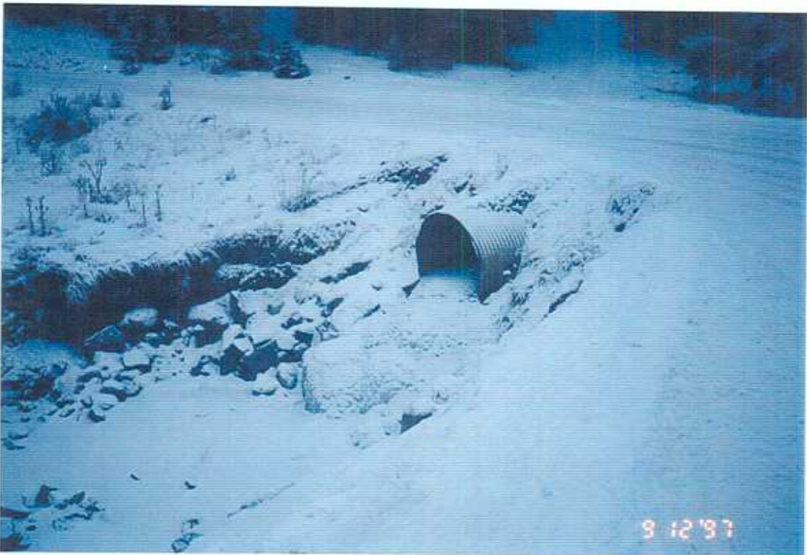
Plate 10: (Site 5) Perched culvert on Tunkwa Creek along Tunkwa Lake Road; erosion occurred downstream of culvert in 1997 (December 9, 1997)
