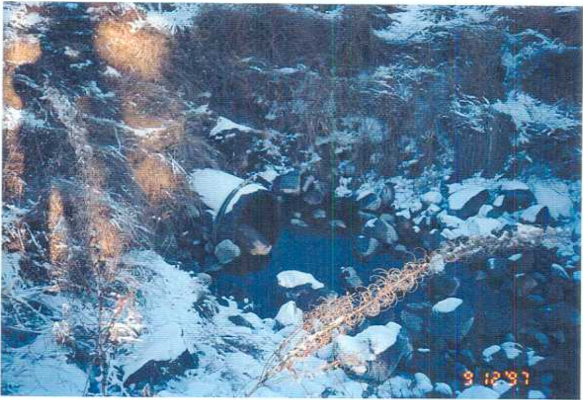
Plate 9: (Site 4) Culvert on Leighton Lake downstream of dam to control water flow into Tunkwa Creek (December 9, 1997)
