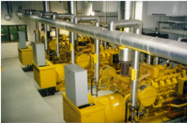
FIGURE D2-1 LFG Gas Engine
