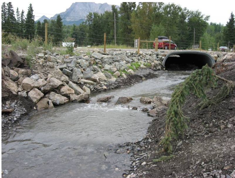
Figure 6: Vortex weir installed approximately 40 m downstream of culvert outlet.
