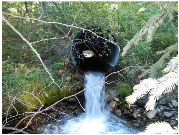
Perched culvert barrel at outlet.
