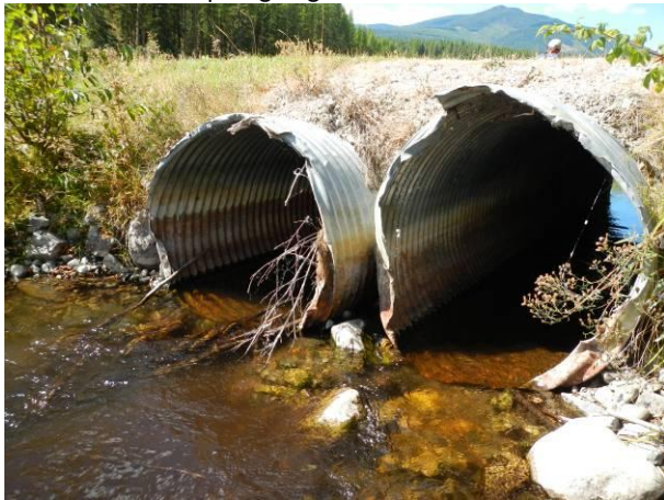
Outlet of culverts. The culverts are not embedded but they are not barriers to fish due to the low water velocity.
