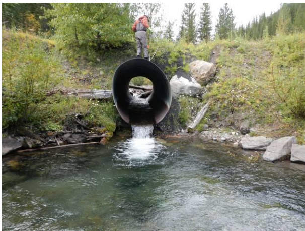
Perched culvert at outlet.
