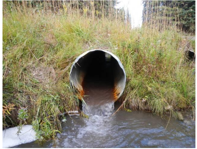
Outlet of right downstream culvert. This culvert is perched but the left downstream culvert is not perched.
