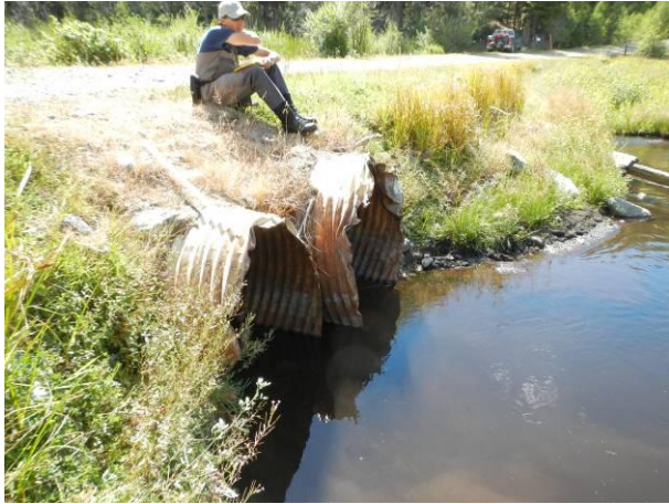
Inlet of culverts. Scour on the road surface indicates that the culverts are undersized and cannot accommodate spring high flows.
