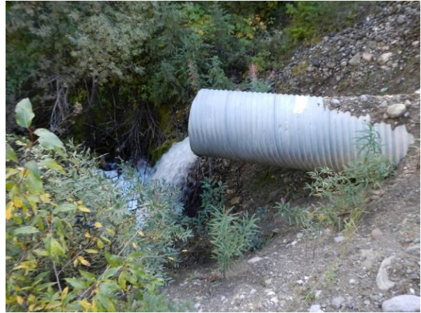
Perched culvert outlet.
