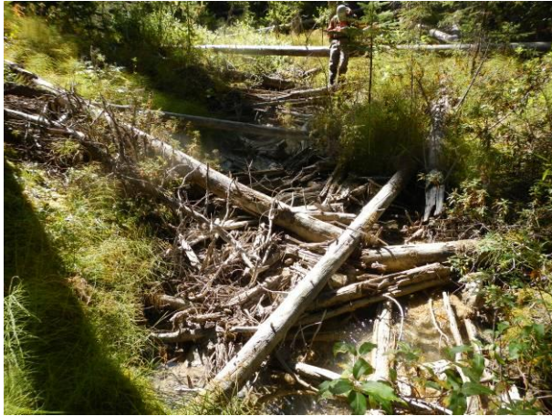
Upstream of culvert. Abundant large woody debris and sediment are present in the stream.
