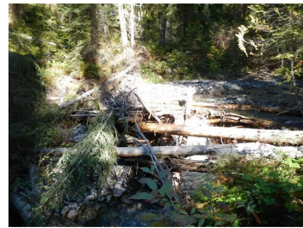
Barrier to fish passage (1.20 m high) created by persistent debris downstream of culvert.
