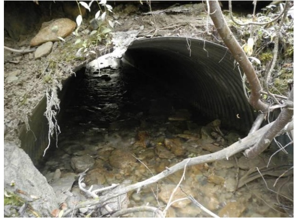
Culvert is partially embedded at the inlet.
