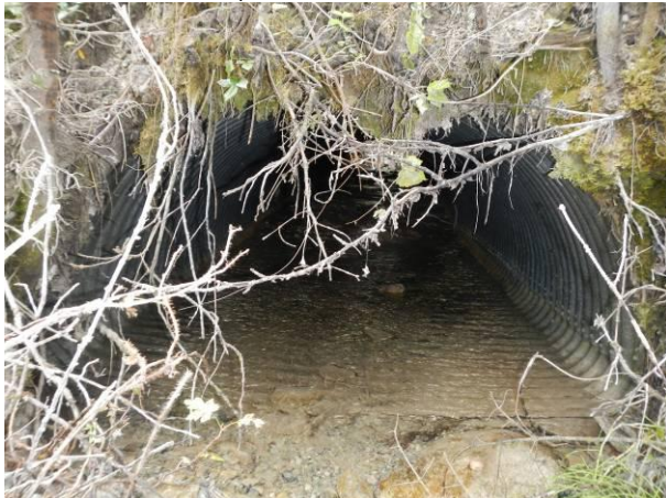
Outlet of culverts. Road fill is spilling over the culvert and covering the outlet.
