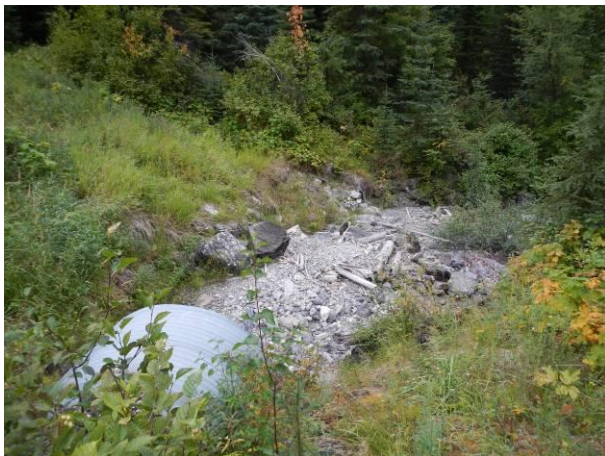
Downstream of outlet of White19.
