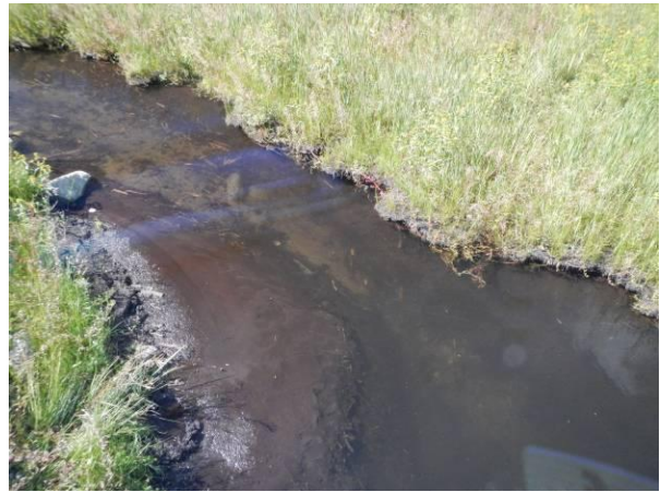
Organic material and silt substrate downstream of culvert.
