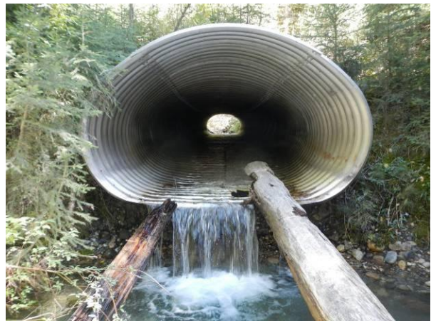
Perched culvert barrel at outlet.
