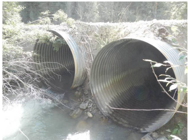
Outlet of culvert. Note that right downstream culvert is perched.
