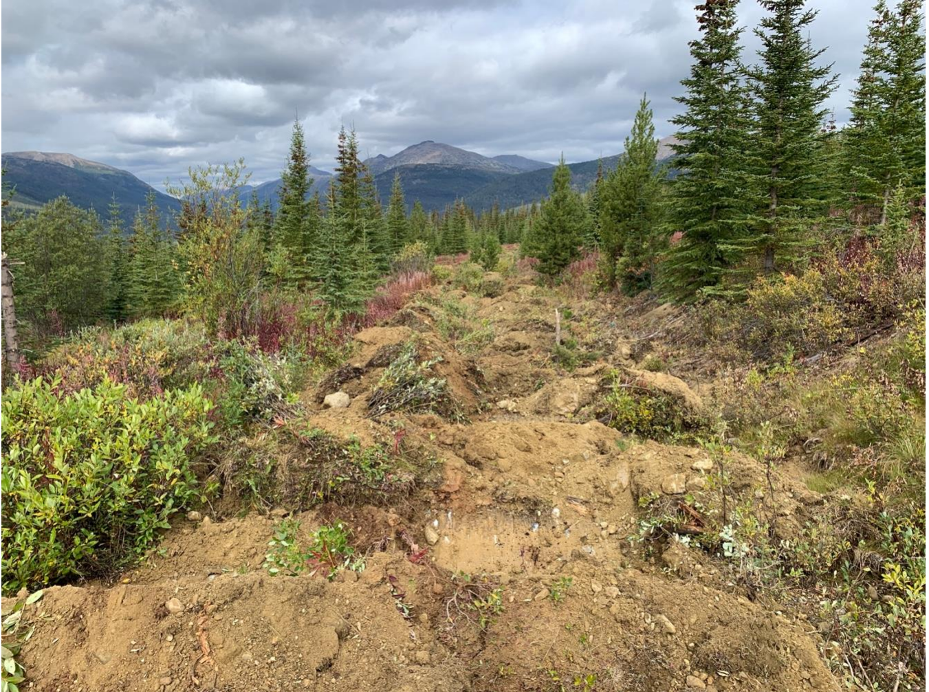
Figure 16. The excavator de-compacted the road surface and the digging bucket was used to create mounds and depressions (pictured above), as well as deep cross ditching and berms for access management. These Mechanical Site Treatments improve soil infiltration capacity, reduce soil bulk density, and create microsites where seeds and planted species can more easily establish.
