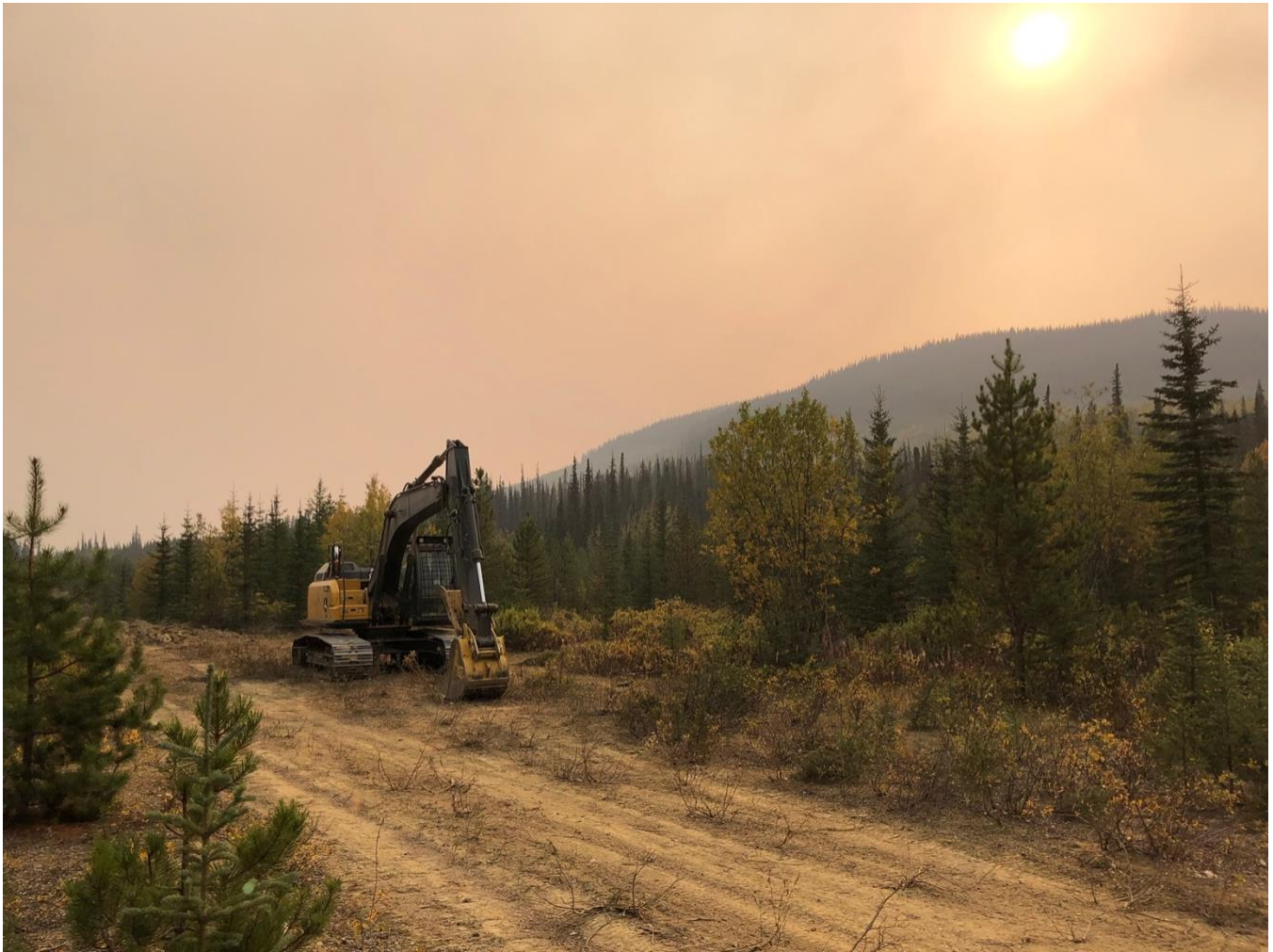
Figure 15. An excavator was used to implement ecological and functional restoration of the Chuyaza road. Pictured is the excavator at the end of a day, with treated road behind it and pre-treatment road in front of it.
