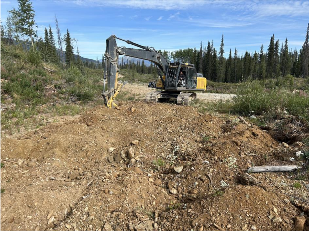
Figure 5.2: The John Deere 210G excavator completing road decompaction and recontouring on a section of road in 2024.
