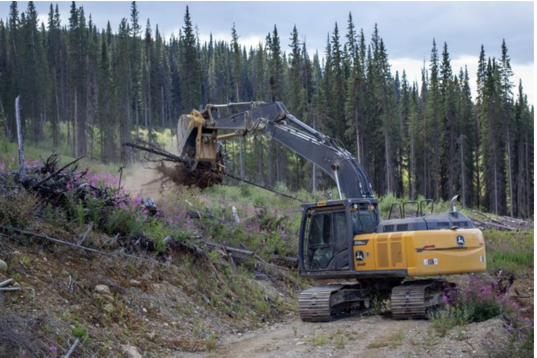
Figure 8.7. An example of the excavator completing slash rollback on a segment of road.
