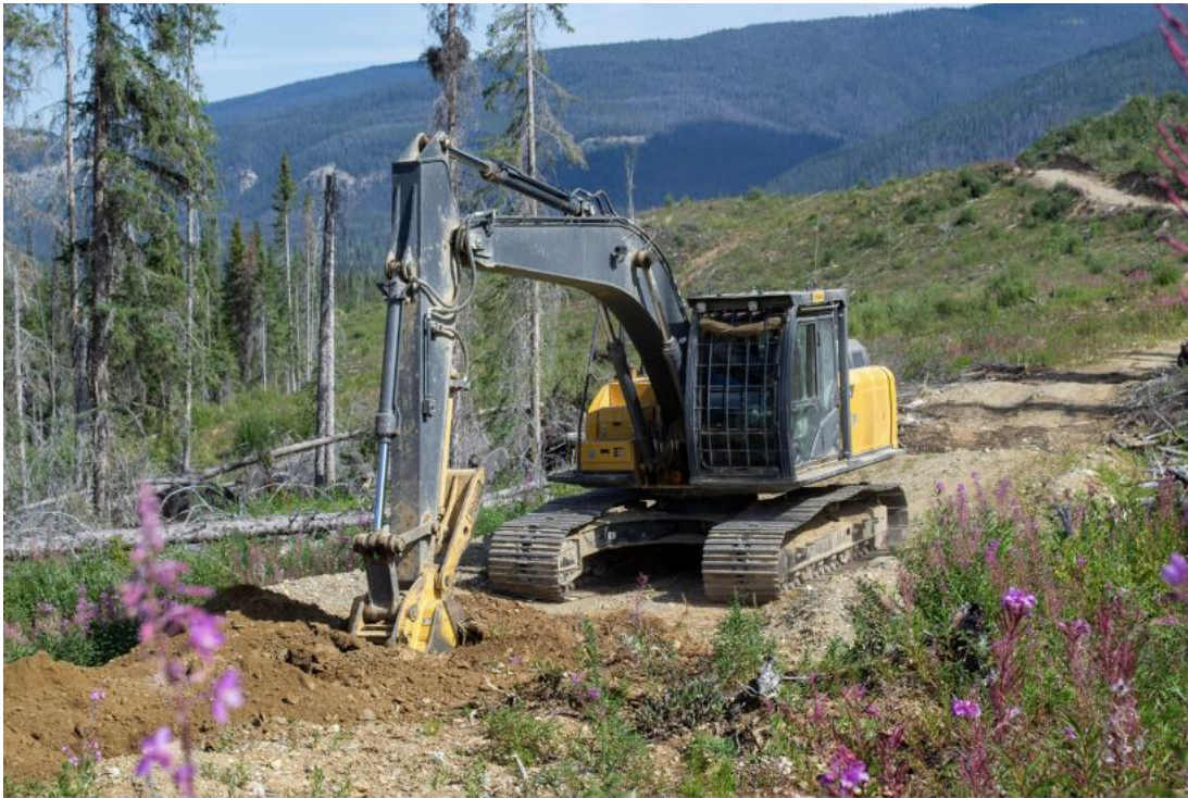
Figure 8.5. The 609 excavator used to implement ecological and functional restoration of the Chuyaza road section: part II. Pictured is the excavator de-compacting and mounding a section of road.
