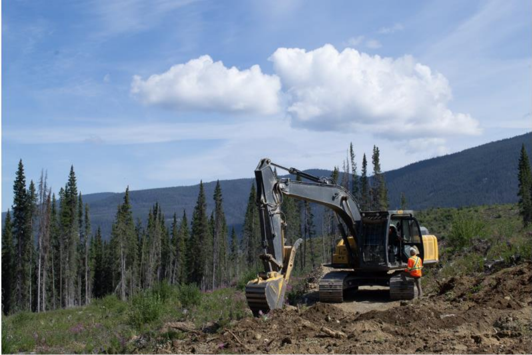
Figure 8.6. The CCE restoration supervisor speaking with the excavator operator about the strategy for the next road segment.
