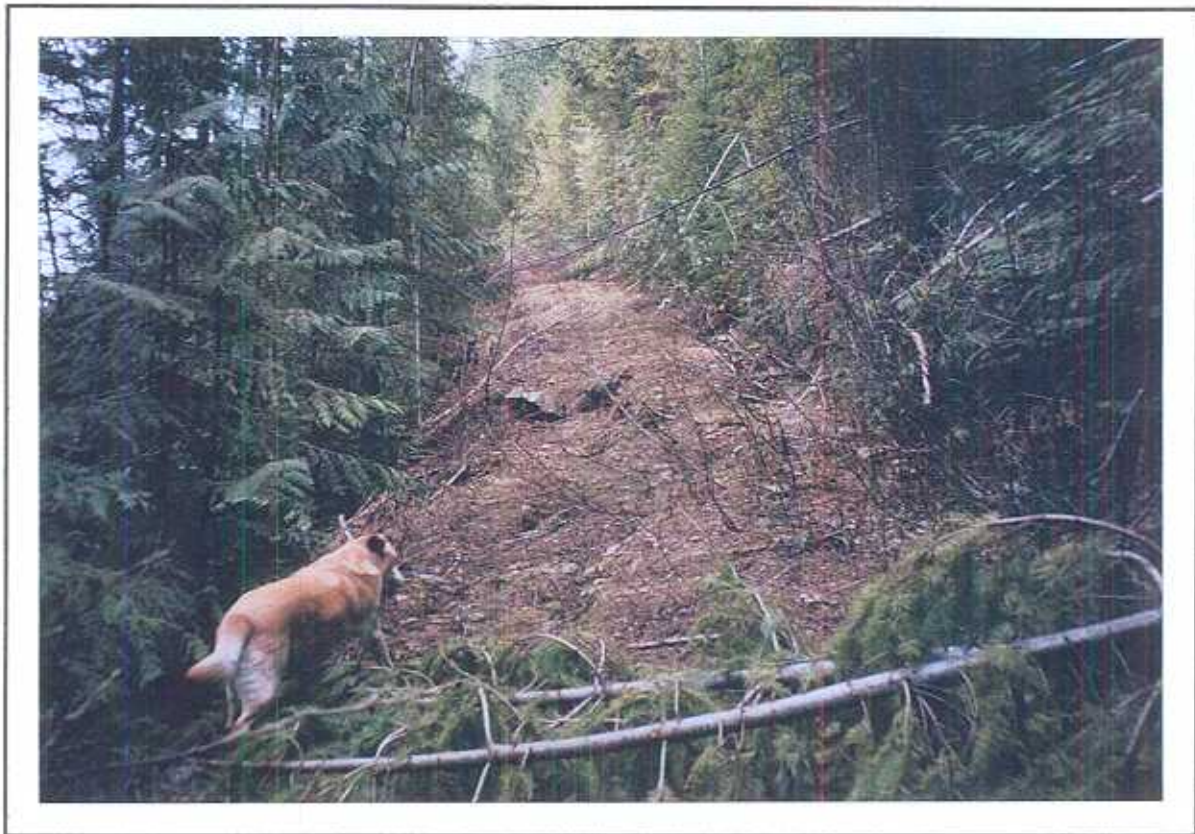
Photo 12. Old tension cracks with fillslope displacement on lower slope road shown in photo 11. Slope gradient is 90% in this location. Similar conditions exist along most of the lower slope road on both side of the East Tributary valley.
