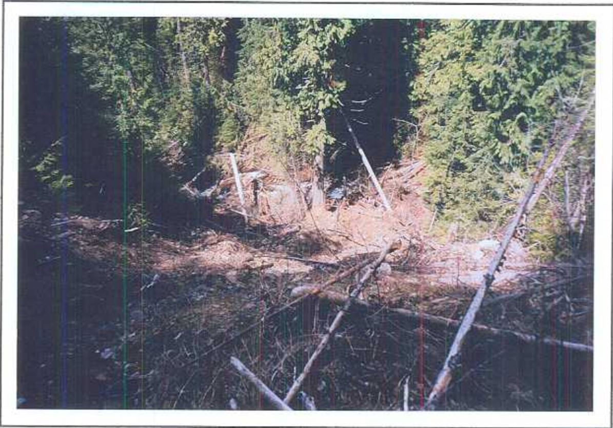
Photo 10. Recent (2001) road fillslope related landslide into reach ET2. Landslide material deposited within 50 m of the impact location and no debris flow was initiated.
