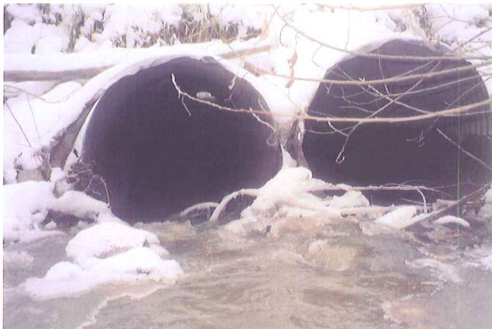
View of inlets
