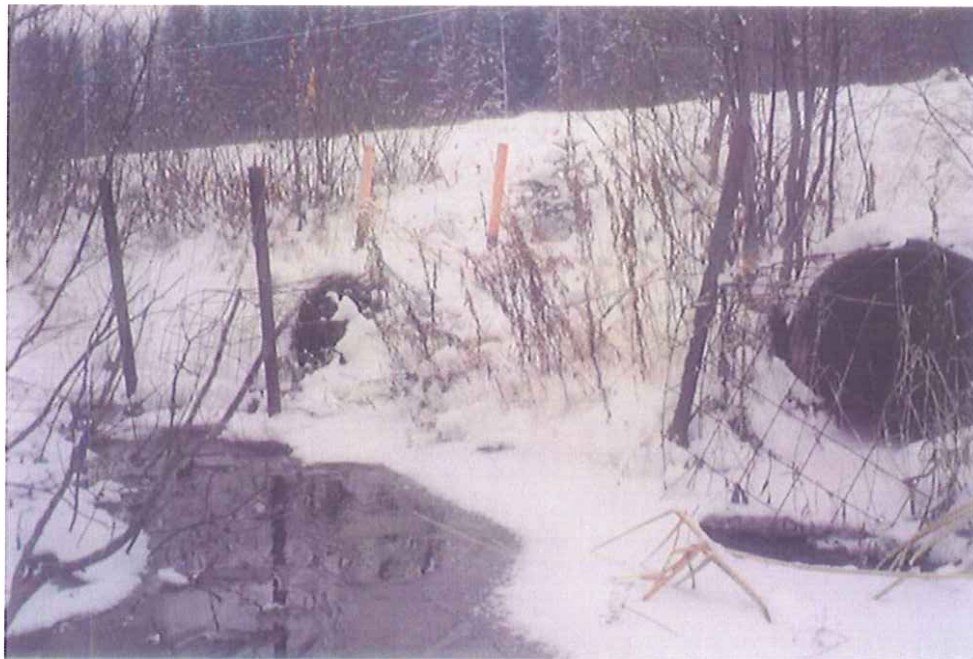
View of inlets.
