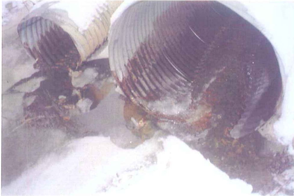
View of inlets.
