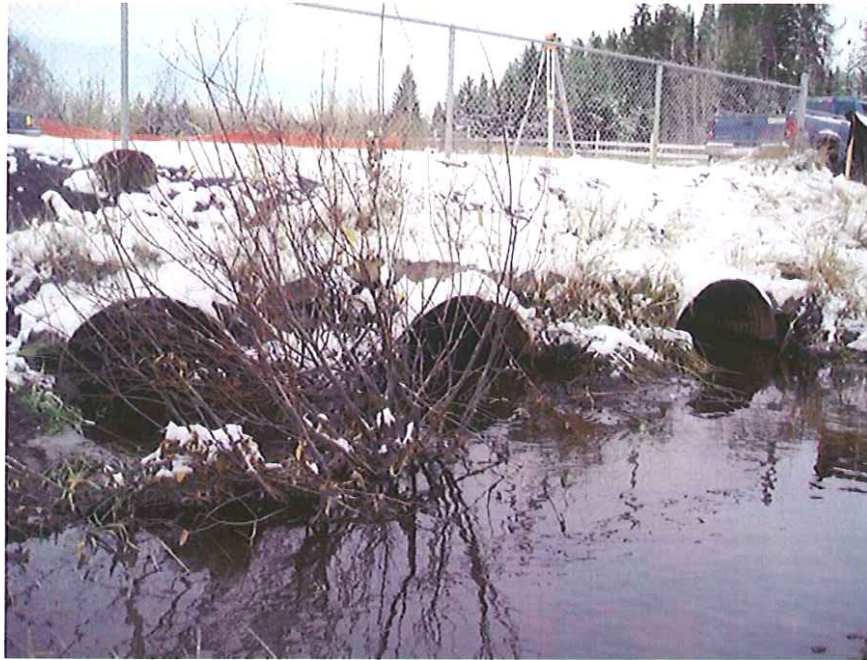
View of inlets.
