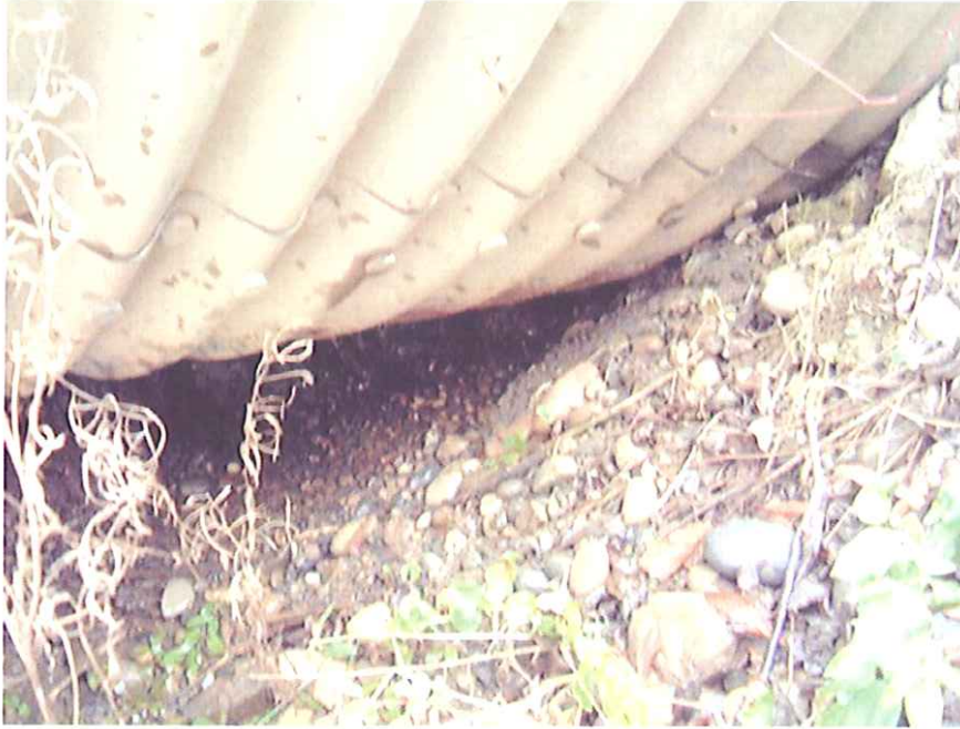
View of outlet. Note the water flowing under the culvert.
