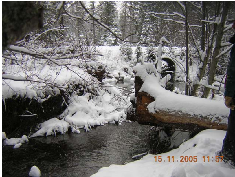
Photo 3 – View looking upstream at scoured channel, uprooted tree and culvert outlet.
