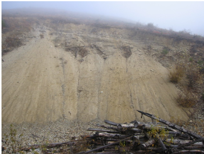
Photo 15. Large cutslope failure in deep glaciofluvial deposits, located in the northeastern portion of the Albreda project area.
