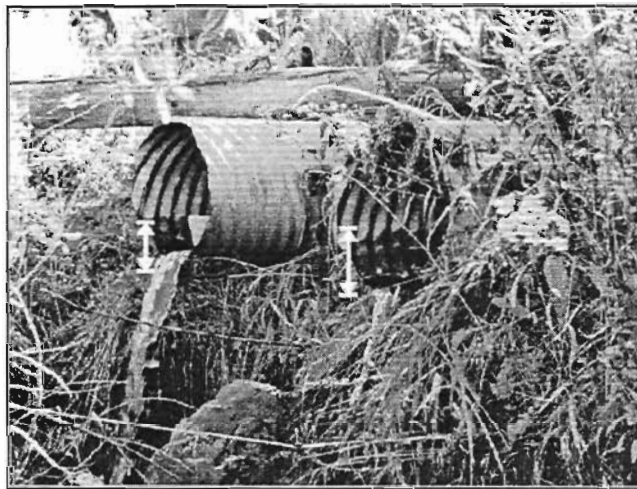
Figure 4. Rust stains on these dual culverts in the Swift River watershed show a high water mark.
