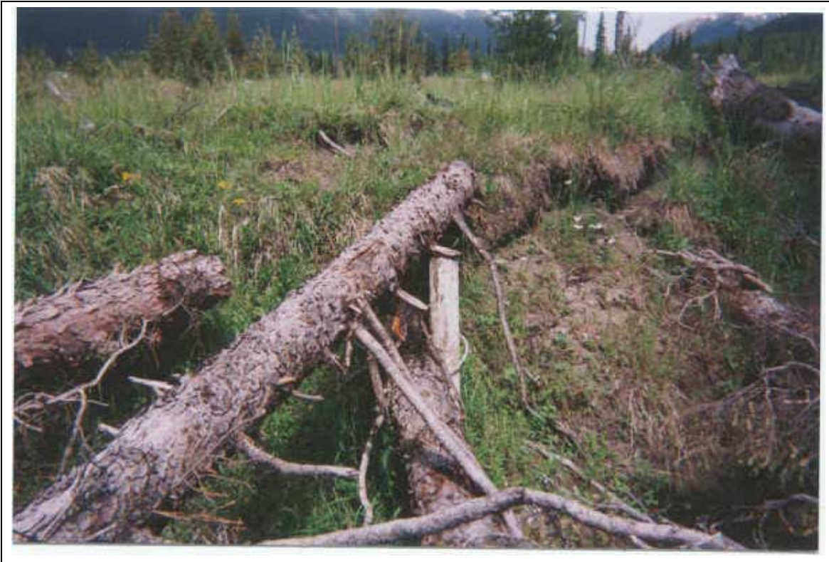
Plate 19 View of typical fence post anchoring used throughout structure, site MY-01, Mayuik Creek (July 22, 2000).
