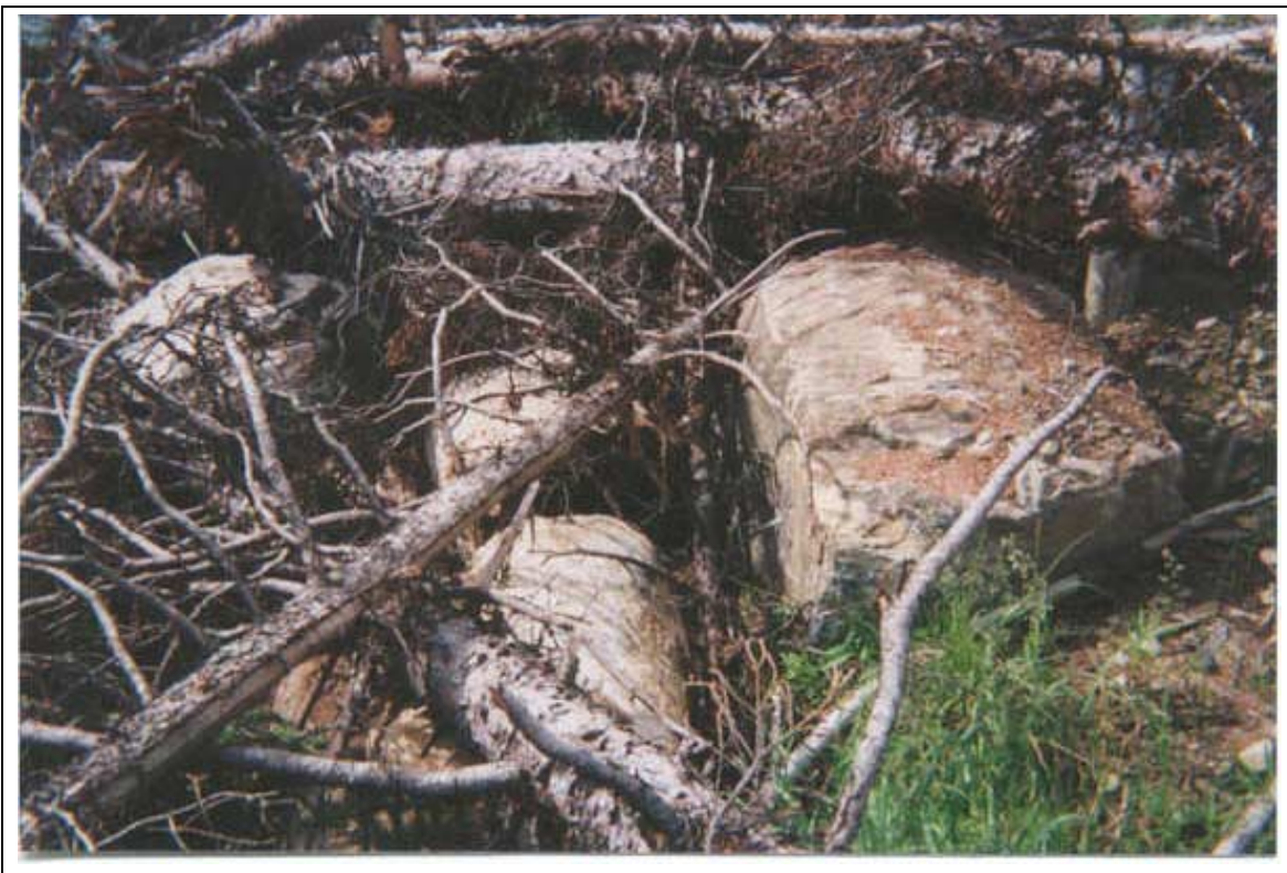
Plate 18 View of boulders used for ballast, upstream end of structure. Site MY-01, Mayuik Creek (July 22, 2000).
