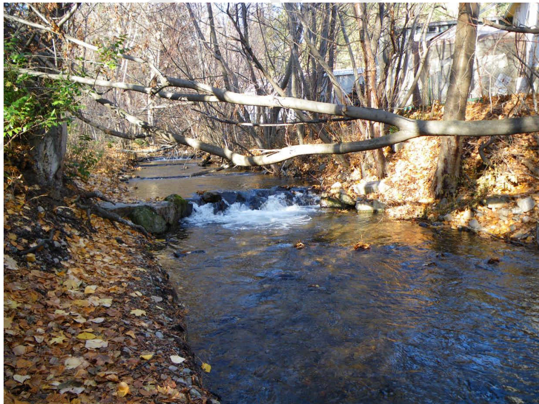
Photo 8. Constructed riffles to improve stability and spawning habitat on Peachland Creek fan.
