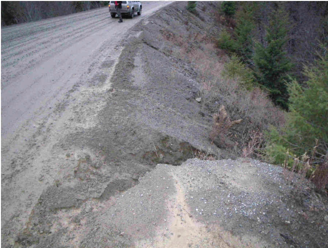
Photo 6. Rill erosion on Peachland FSR fill at Peachland Creek crossing.
