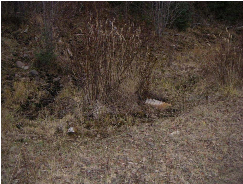
Photo 8. Example of cattle related damage to drainage infrastructure in Tranquille basin. Diversion of flow from this site has scoured an erodable ditchline with input to Tranquille River.
