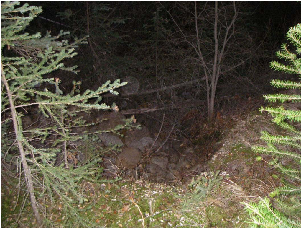
Photo 17. Erosion on steep coupled slope downstream of culvert shown above. The site is connected to Tranquille River.
