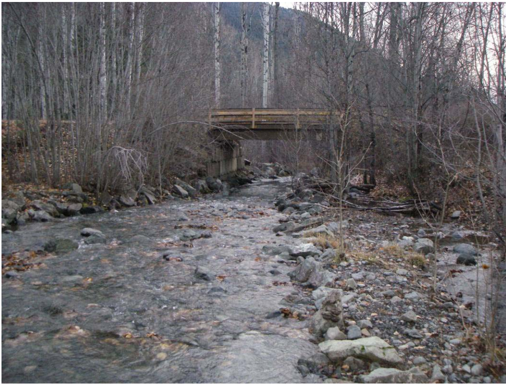
Photo 4. Sawmill FSR crossing on Watching Creek floodplain. The active floodplain is constricted by the structure – sediment and debris accumulation at the inlet is likely during high flow periods. A washout could affect public safety, public infrastructure, access, and water quality.
