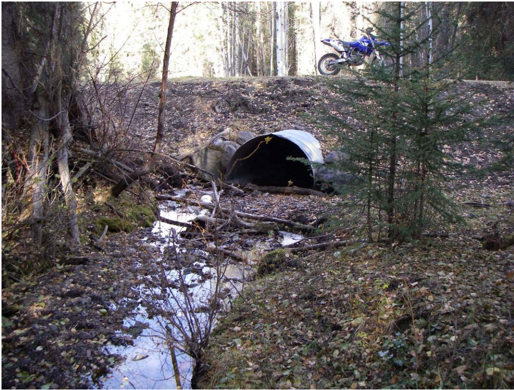
Photo 15. Mobile sediment and debris accumulation at road 4030.25 crossing on alluvial fan.
