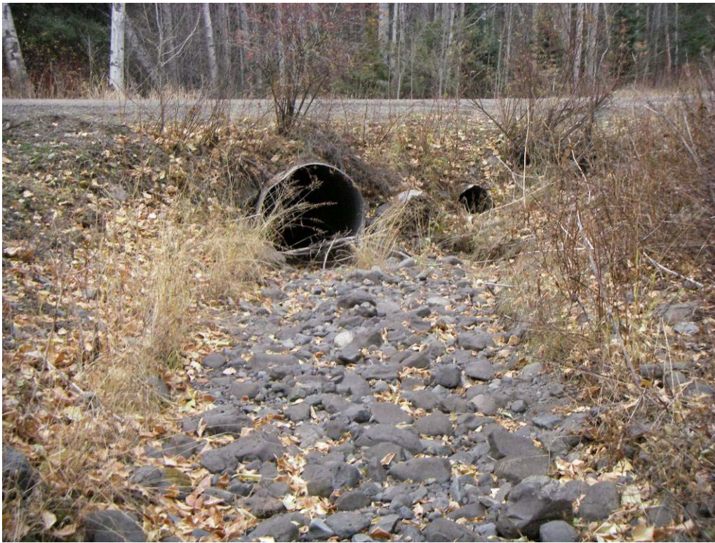
Photo 13. Undersized culverts on Red Lake road at Sylvestre Creek crossing. The channel is active on the fan; structures have failed at least once already causing diversion down the ditchline with flow over the road. This site was identified as a problem by Summit in 2003.
