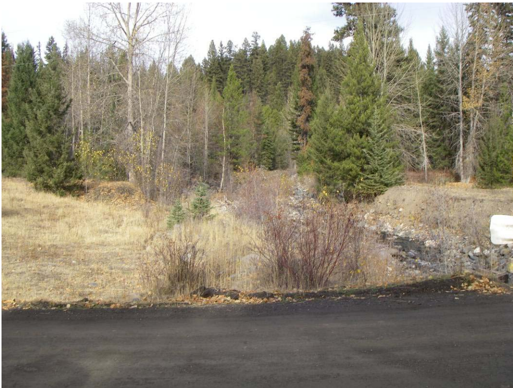
Photo 10. Red Lake road crossing near toe of fan shown in photo above. The structure is undersized and will fail during high flow events that result in sediment and debris accumulation on the upstream side.
