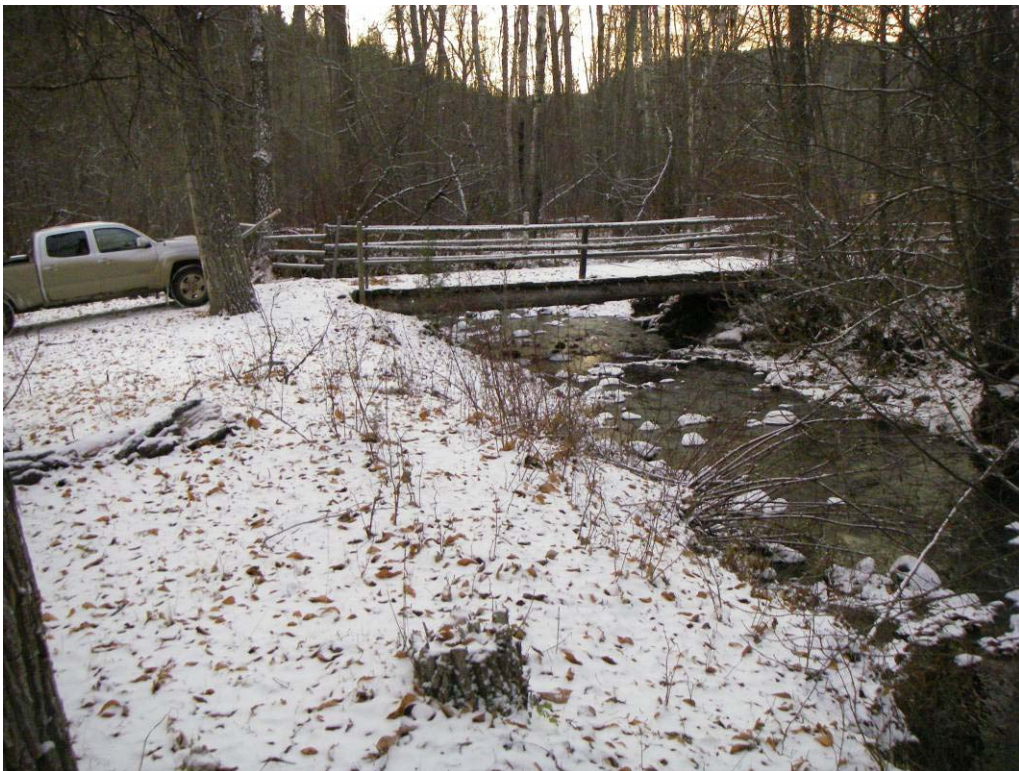
Photo 5. Non-status road crossing on Watching Creek downstream of Sawmill FSR. The structure is on the active floodplain and will likely fail during high flow events that mobilize upstream sediment and debris.
