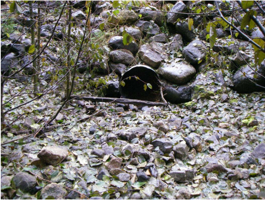
Photo 10. Brendan Road crossing on large S6 channel in residual with mobile sediment and debris. Culverts on channels like this are prone to failure as a result of sediment and debris accumulations at the inlet. Oversized culverts or open bottom structures are more appropriate in these cases.
