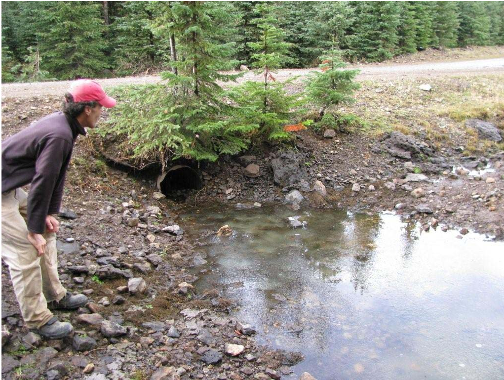
Photo 8. Blocked culvert at Home FSR crossing on Home Creek. Flow is diverted down the ditch from this site and into the Mosquito basin where increased discharge is scouring channels, increasing sedimentation levels, and stressing downstream road infrastructure.
