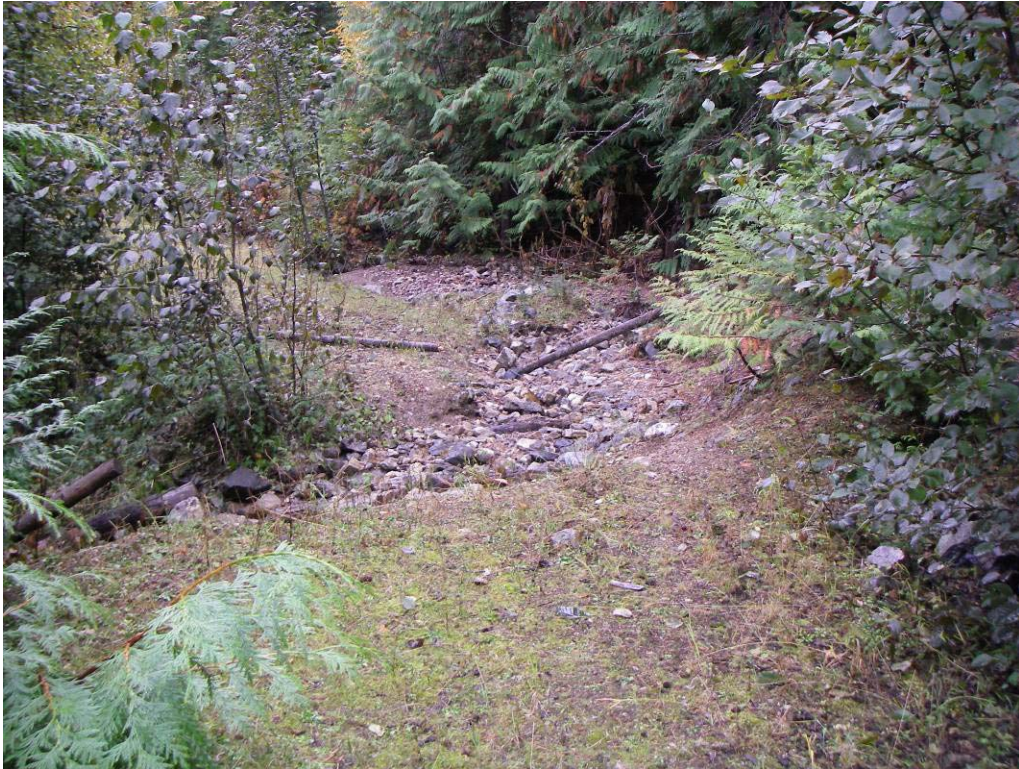
Photo 11. Failed culvert at Upper Amy non-status road crossing on tributary in residual. Flow is moving through waterbar but diversion down the road is likely with ongoing erosion and both range and recreational use.
