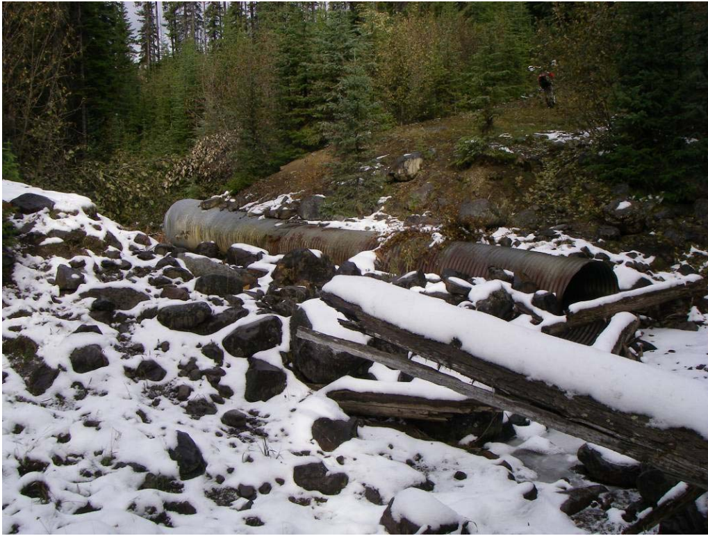
Photo 12. Washed out H100 non-status road crossing on Upper Harris tributary. The site is a source of sediment to fish bearing waters, a barrier to fish passage, and eligible for deactivation using FIA funds.
