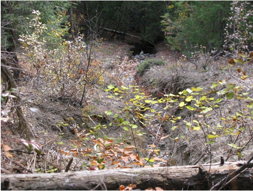
Photo 4. Erosion in glacio-fluvial terrace materials below culverts on Jeffery and South Jeffery Roads. Drainage is diverted and concentrated on these sites from roads leading down to or built on the terrace.
