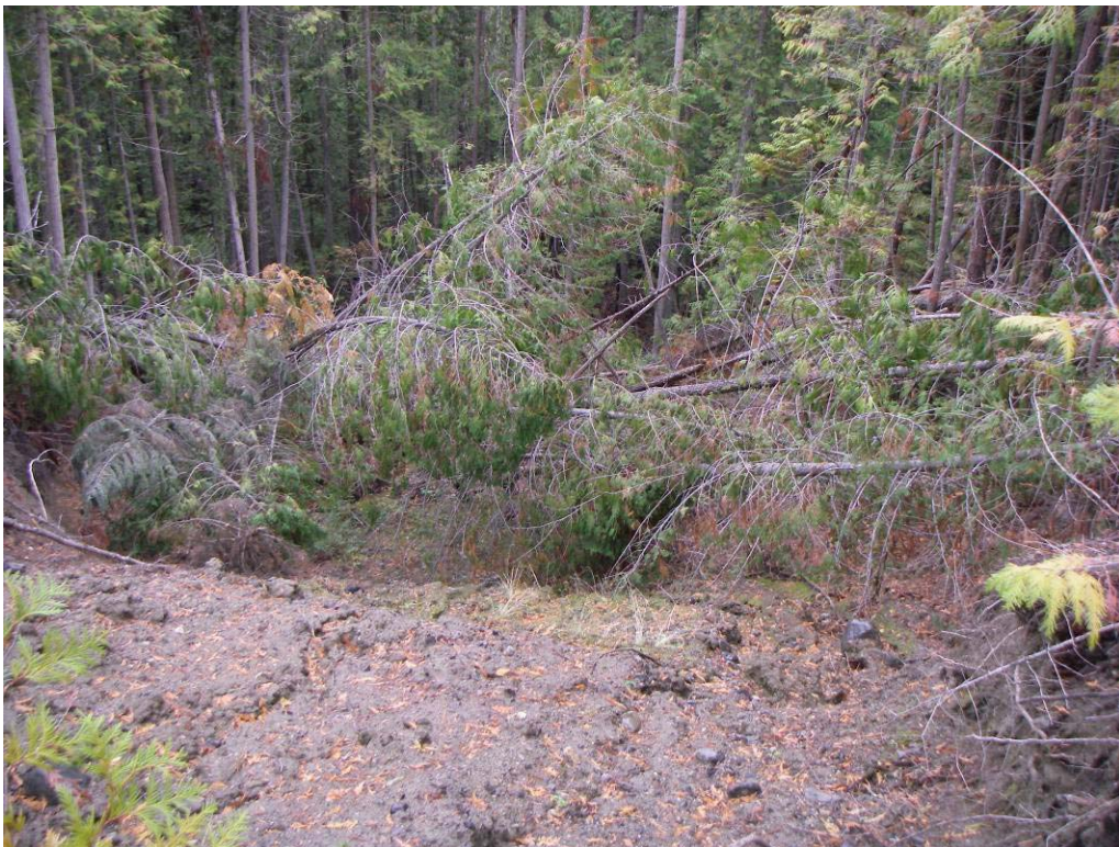
Photo 2. Recent landslide off of Harris Southwest non-status road from culvert discharge on Dustin Road above.
