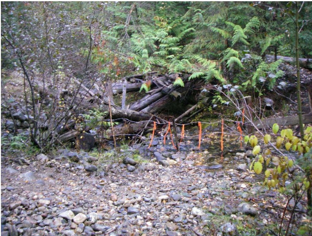
Photo 7. Failed Denis non-status road crossing on McAuley Creek floodplain. Approaches are built from alluvial material, are restricting floodplain processes, and will continue to erode over time with input to the channel.
