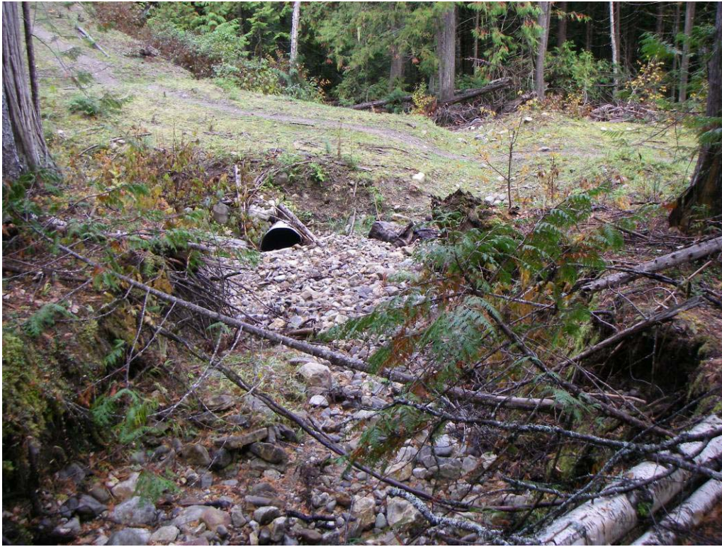
Photo 6. Scoured fan channel and infilled culvert on Dustin F road. The structure is backed up with a water bar but not armoured. The road prism will washout when the structure fails and flow may escape down the road to the southwest. Downstream of the crossing the stream has diverted down the Harris Southwest non-status road resulting in significant scour and sediment input to Harris Creek. Situation typical of road crossings on fan.
