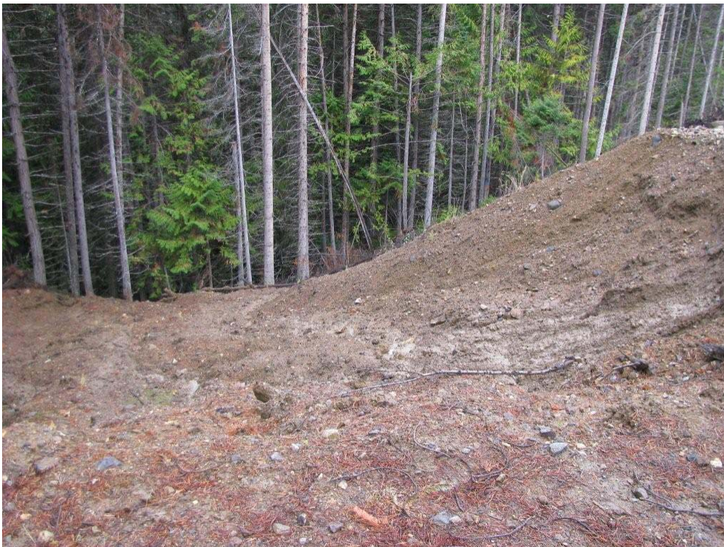
Photo 9. Recent slump off of upper switchback on Dustin Road above West Harris Creek. Cutslopes and drainage infrastructure are failing in this area resulting in drainage diversion onto Class IV terrain.
