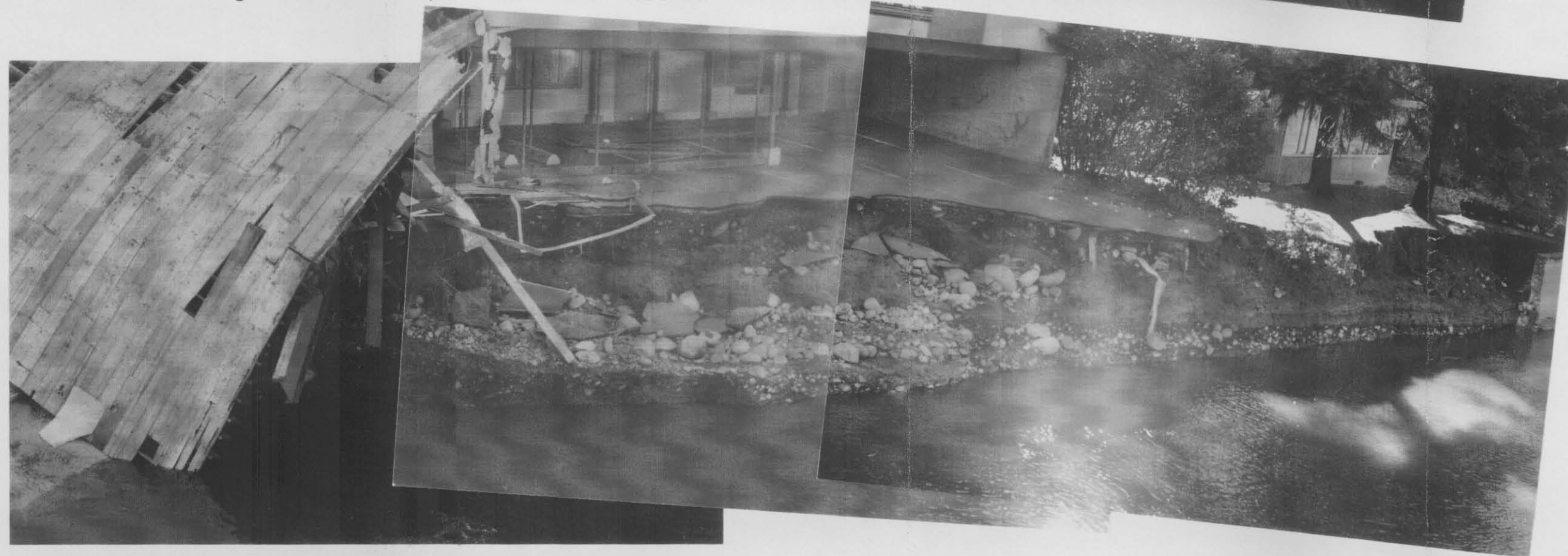
8. Panorama showing severe erosion and subsequent structural damage on the left (east) bank downstream of the Dollarton Highway bridge at XS-5/6 following the October 31, 1981 flood of record.
