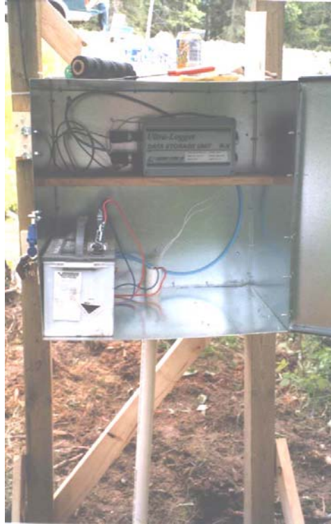
Figure 3.2.2 Hydrometric station located at the Wigwam River Bridge. Metal housing was used to protect the data logger that recorded water level, temperature, air temperature, and precipitation every 15 minutes.
