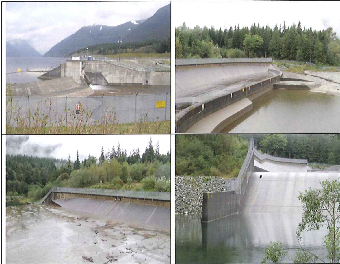
Figure 4. Alouette Spillway Top: free spill crest and crest gate (left), and free spill crest (right). Bottom: Spillway low gradient section (left) and high gradient section (right).
