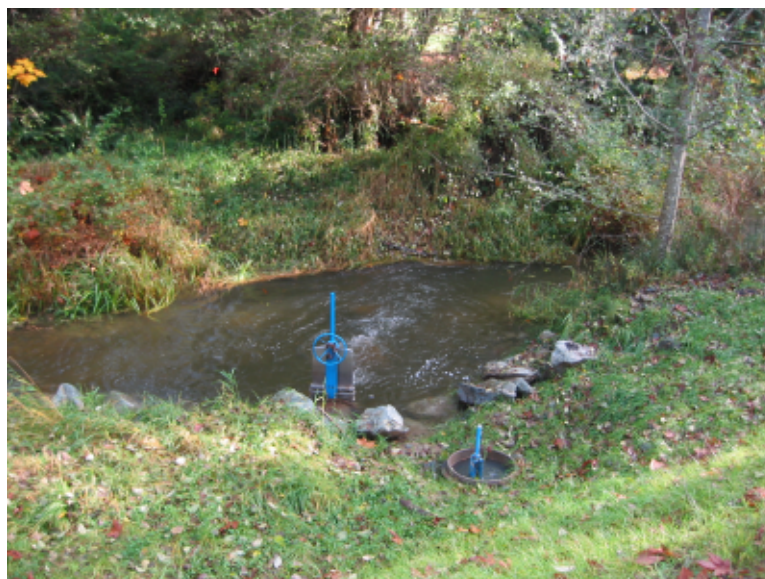
Figure 1 600mm Intake Valve and 300mm Bypass Valve
