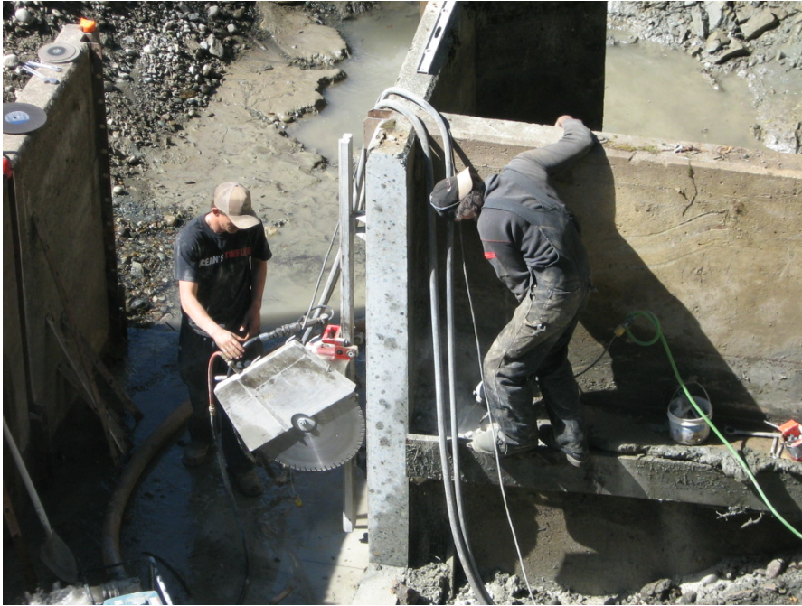
Photo 3. A concrete saw was used to cut the fishway and left bank abutment. An excavator lifted the concrete sections out of the way.
