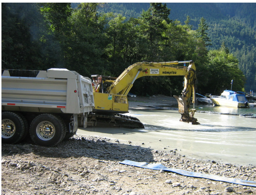
Photo 8. The area upstream of the weir was isolated and a low flow channel was excavated connecting the lake to the weir.
