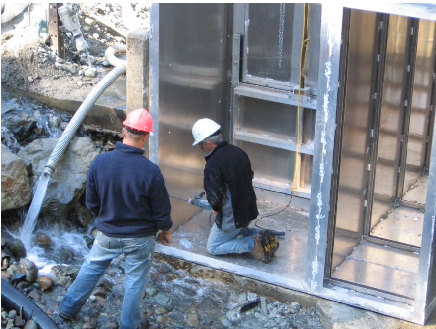
Photo 6. Concrete anchor bolts were used to secure the aluminium fishway to the concrete footings.
