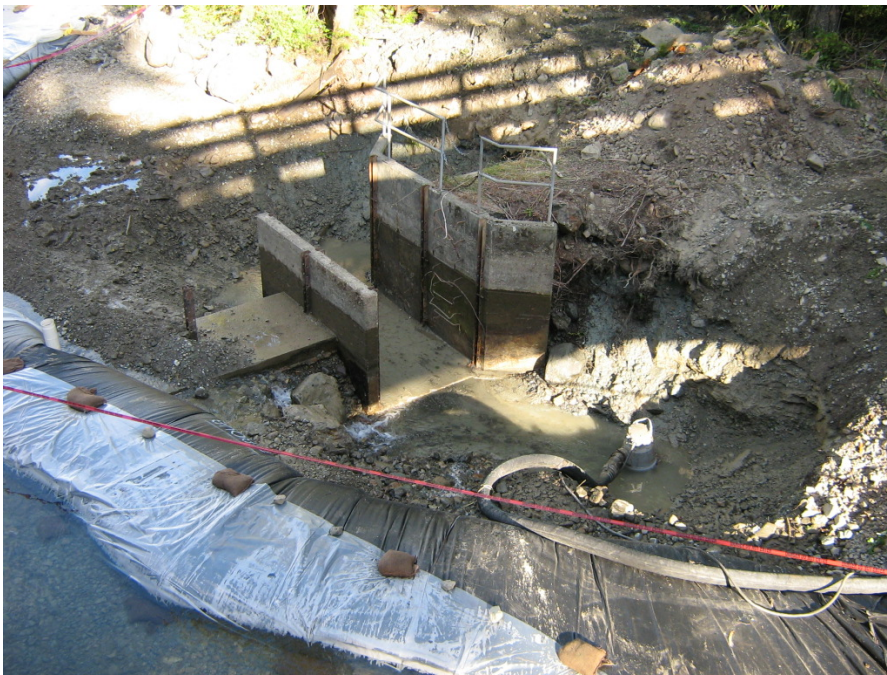
Photo 2. Aquabags and a 600 volt, 150 mm submersible electric pump were used to isolate the fishway area.
