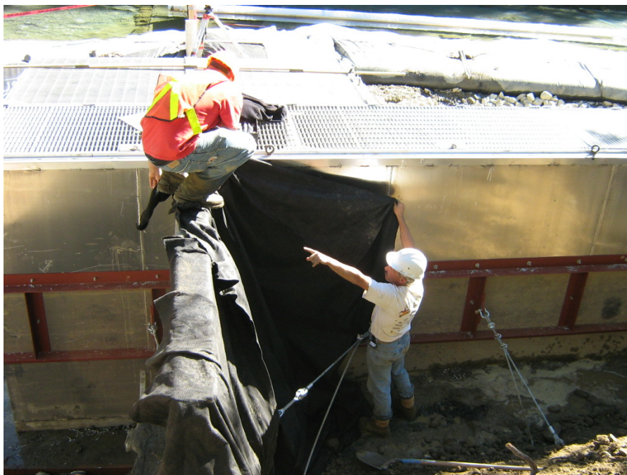
Photo 7. A steel reinforcement ladder was bolted to the side of the fishway. Galvanized steel cables linked the ladder to the concrete abutment and a block buried in the bank.
