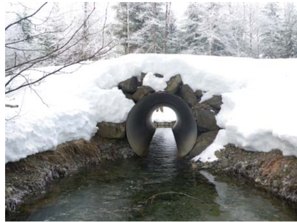
Photo 1. View of 2000 mm CSP at crossing 304 in the Taylor River Watershed, January 2009.
