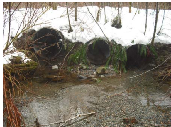
Photo 2. View of the multiple culverts at crossing 87A in the Nitinat River Watershed, February 2009.
