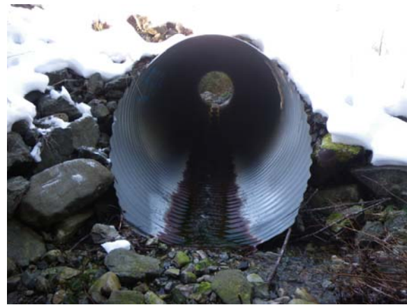
Photo 1. View of 2140 mm CSP at crossing 1335 in the Toquart River Watershed, January 2009.
