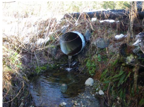
Photo 2. View of the hanging 1000 mm culvert at crossing 2557 in the Toquart River Watershed, February 2009.
