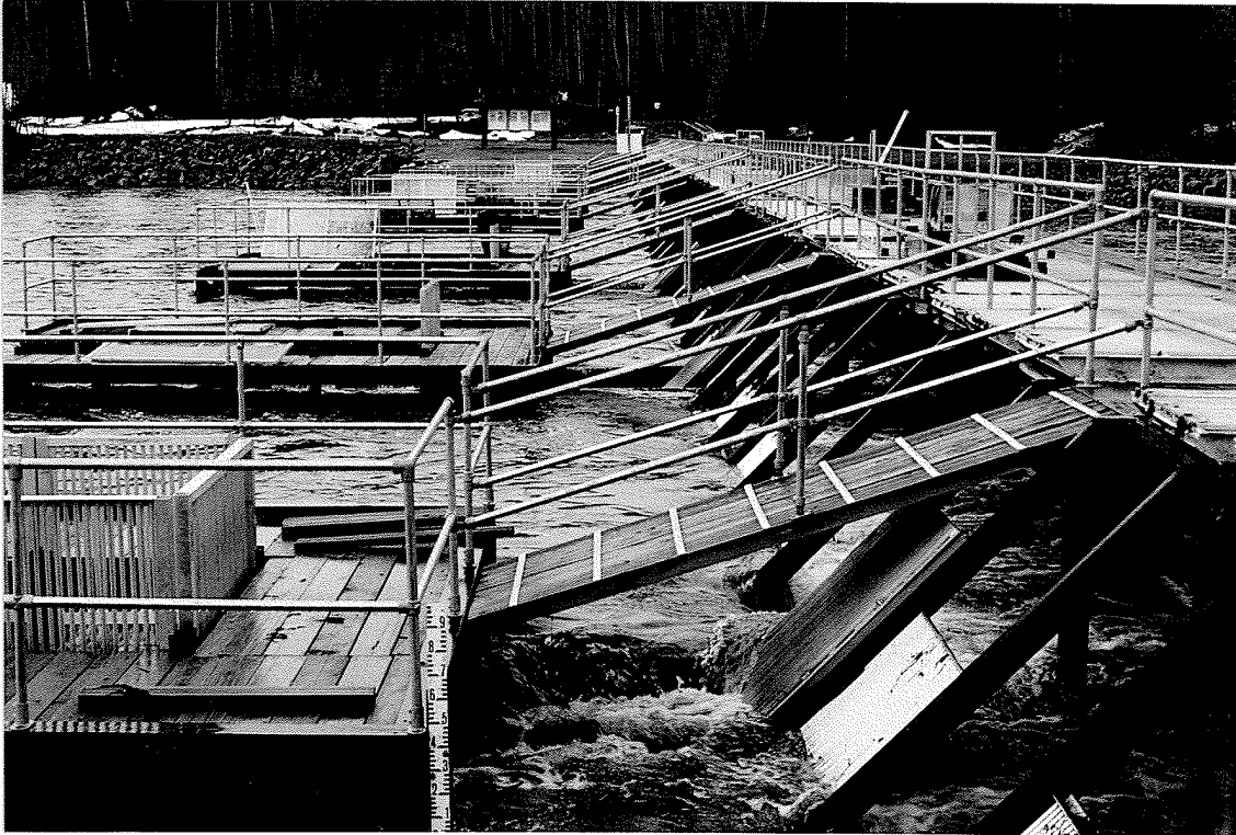
Figure 10. Photograph of fence on May 18 th , when discharge overflowed the new fence panels by approximately 10 cm.
