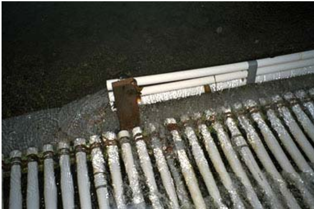
Photo Figure 4. Close-up, showing the baffle raised up off the panel. Note the 2x4 wood and the duct tape holding the P.V.C. pipes together.
