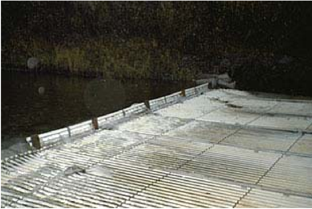
Photo Figure 3. View of low water baffle system. Note the lack of water on top of the panels.
