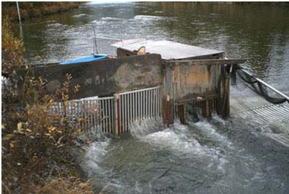
Photo Figure 6. View of downstream end of the fence trap box showing aluminum panels between the trap box and the right bank.
