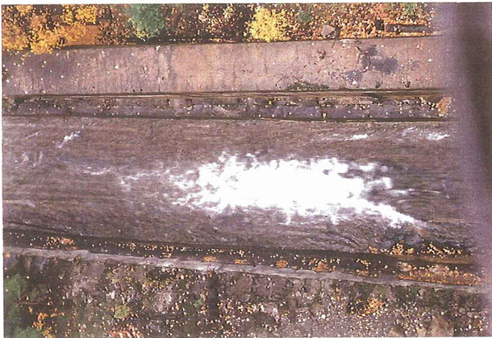
Figure 7. Lower portion of flume under the railway crossing at the top of Kwoiek Creek Reach 1 (viewed from above).
