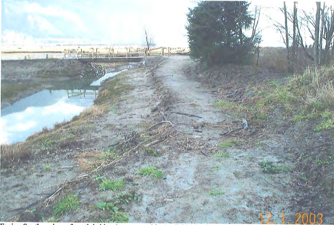
Facing South – view of south bridge (constructed in April 2003) with access to berm/trail to left
