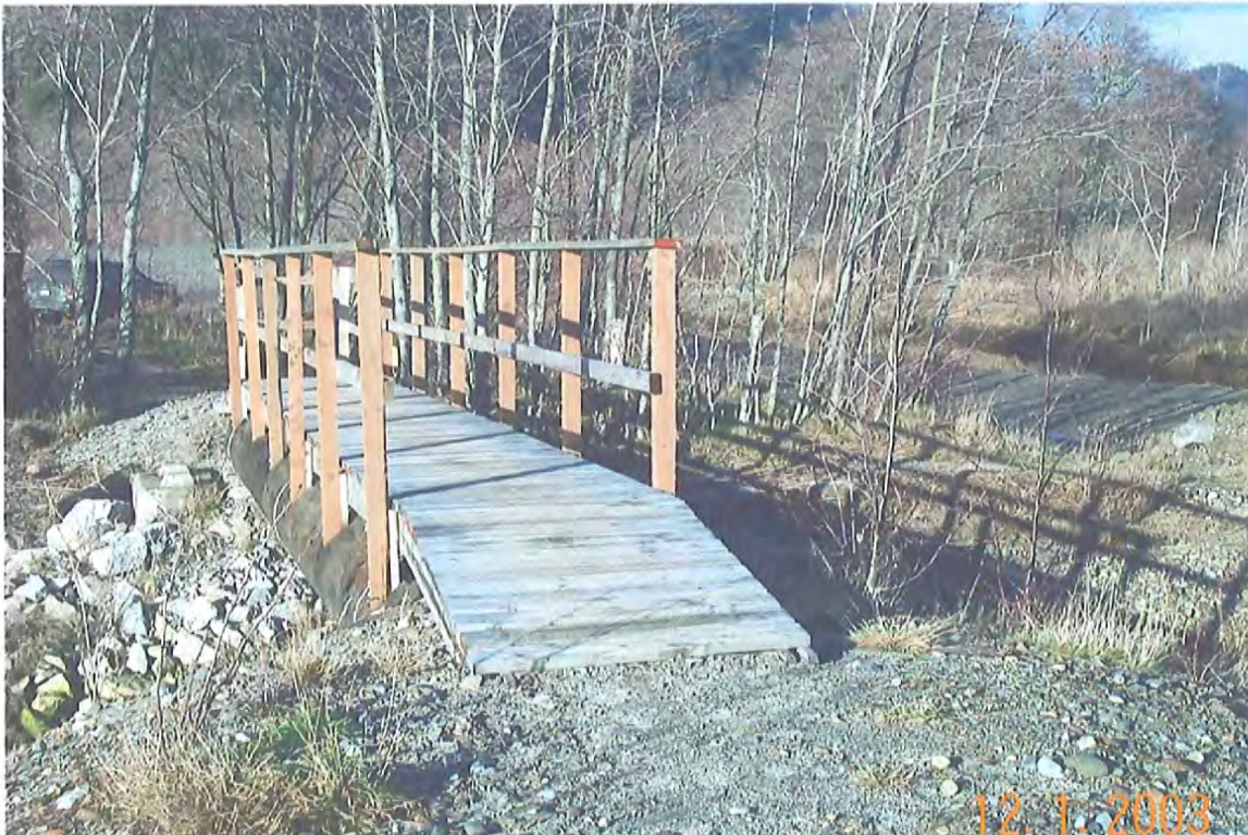
North access bridge across channel (access road/Training Dyke and parking area can be seen in the background – channel from River access can be seen to the right)
