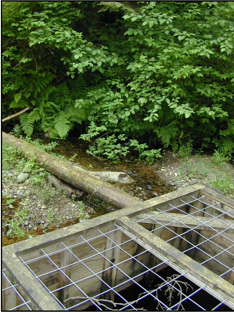
Figure 34. Beaver box and culvert at site HR CU1.
