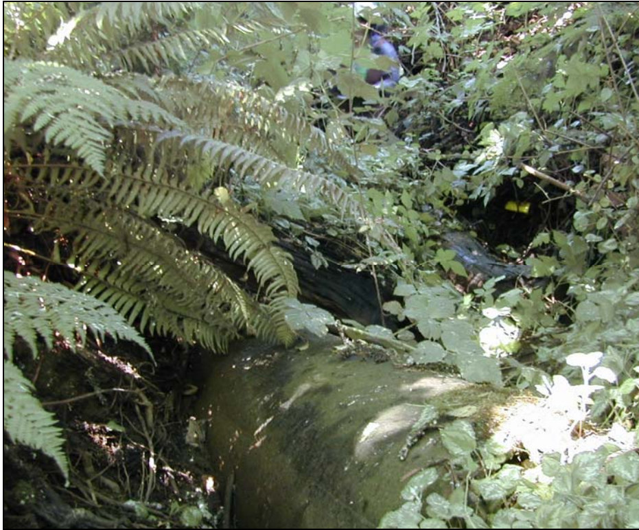
Figure 22. Fragmented instream culvert at site SI 210 on McKinney Creek.
