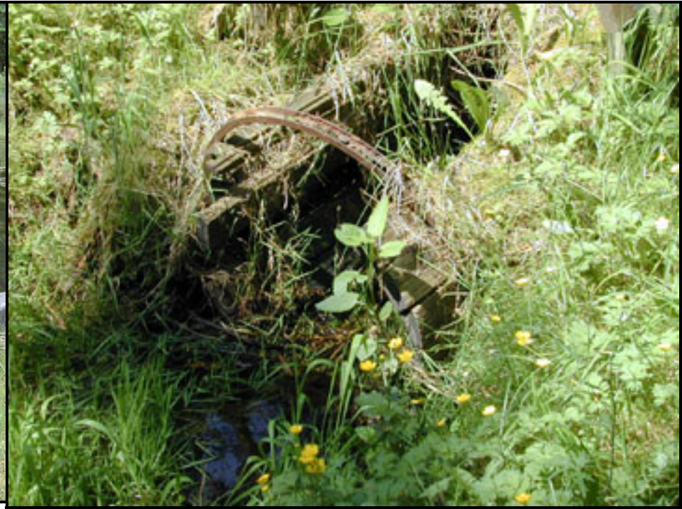
Figure 29. Decayed culvert at site CU 346 on Dogwood Creek.
