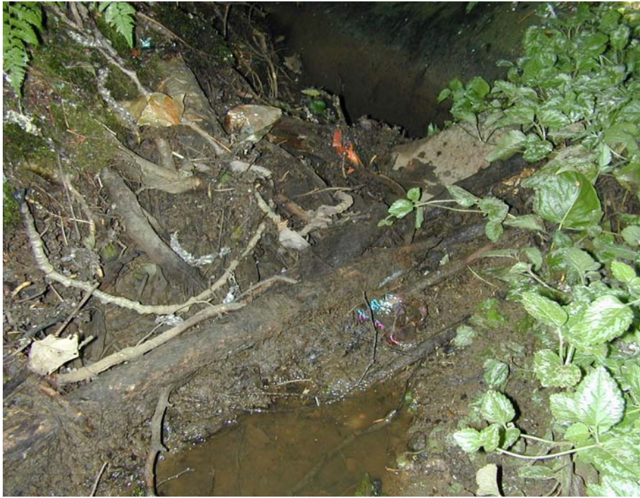
Figure 32. Woody debris and garbage at site NO 240 on McKinney Creek.
