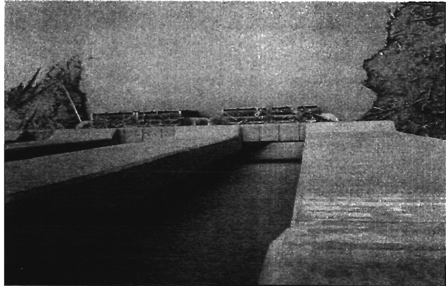
Plate 6 View down the stop log slots illustrating why the trash racks prevented any object from being lowered into the intake from the top of the intake structure. Photo taken April 1996 at a reservoir elevation of 698 masl (BC Hydro photo).
