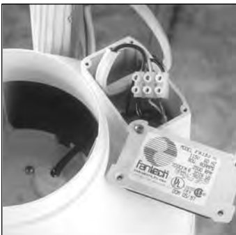
Romex wiring – Top View
