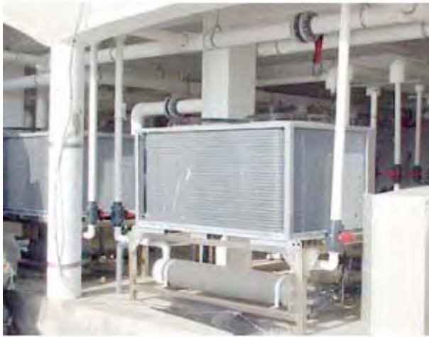
20 HP Water Chiller in Operation.
