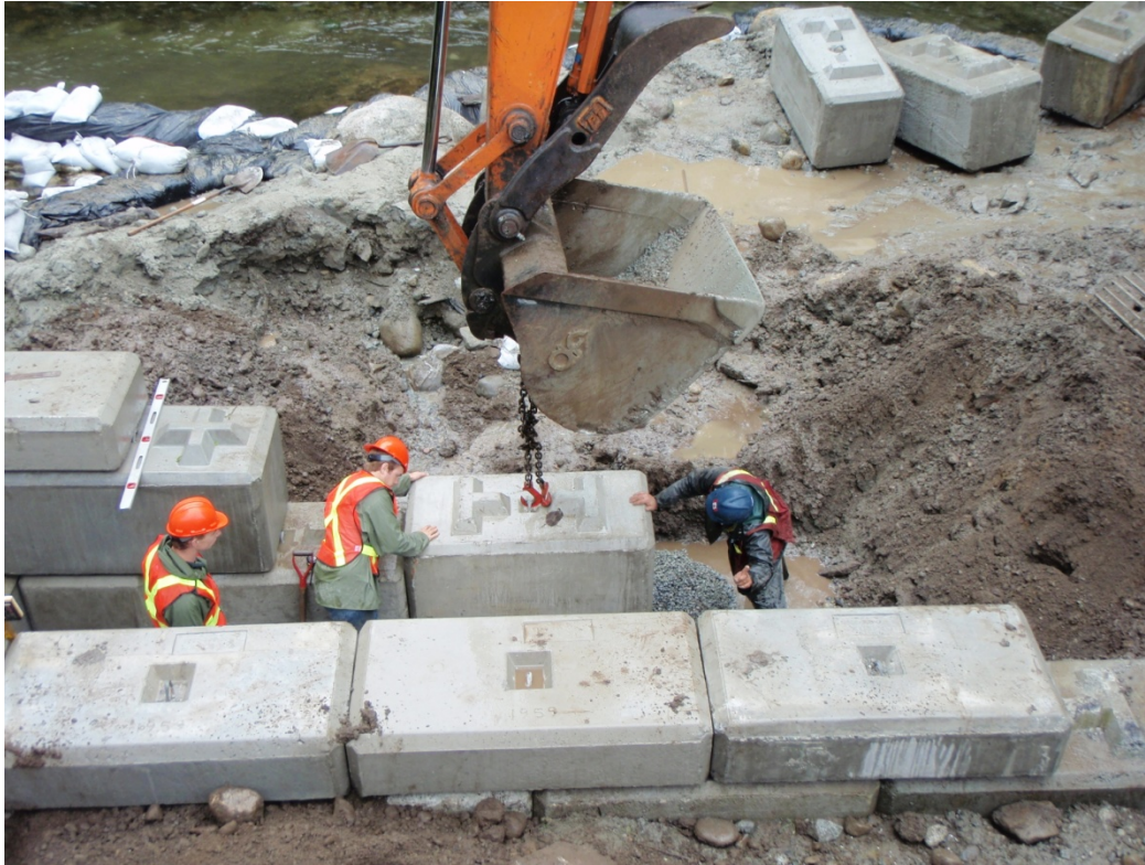
Figure 3: DFO Engineer Technicians place lock-blocks which form the sides of the new trap, 2008.
