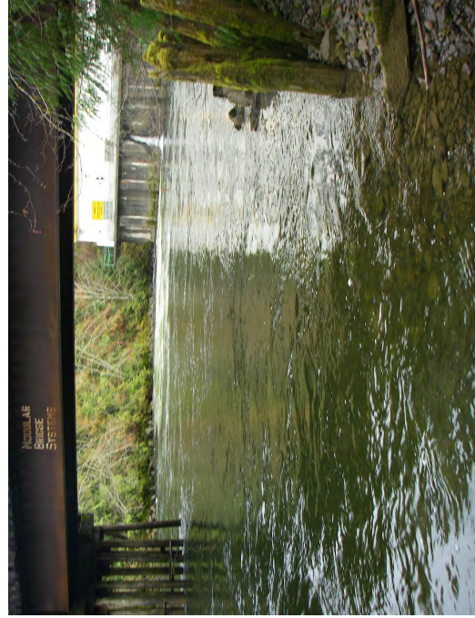
Figure 4: Pilings evident beneath bridge spanning Powerhouse Channel as well as piling remnants from a historical bridge crossing on right and Powerhouse visible in the background.
