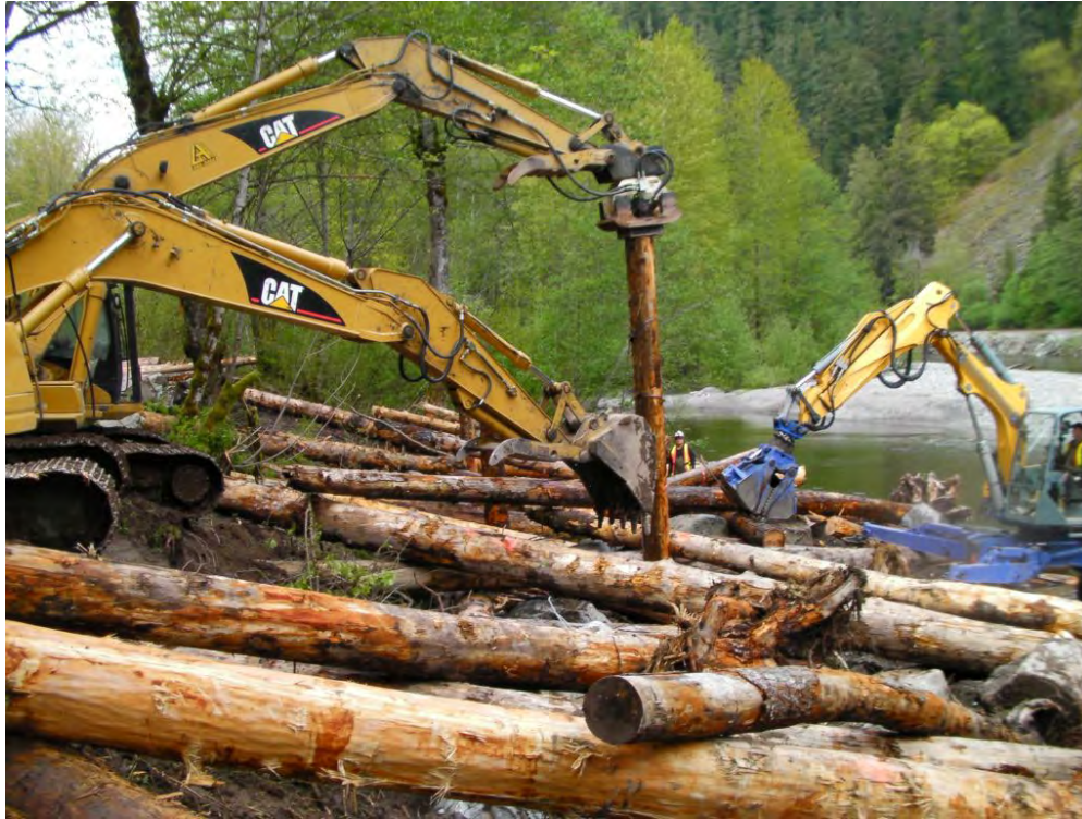
Photo 2. Driving piles using Vibratory Pile Driver attachment at LWD structure site in Cheakamus River, May 2010 (photo credit D. Harper, BCCF).
