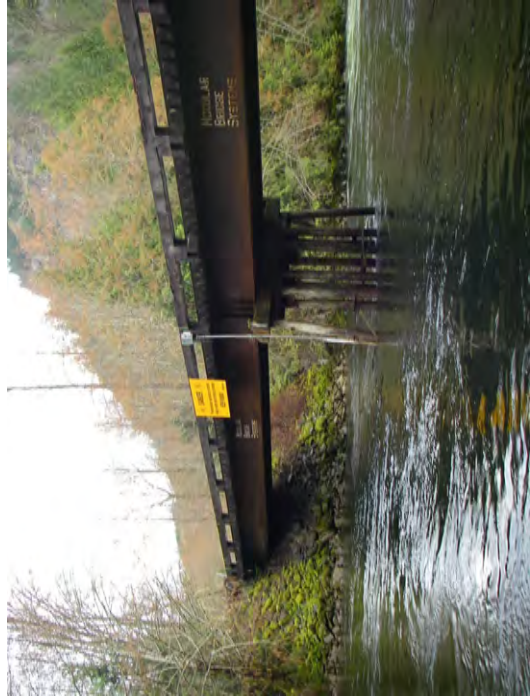
Figure 3: Upstream end of Powerhouse Channel, also the starting point of the field survey performed on March 17, 2010.
