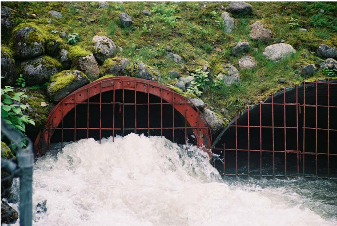
Photo #4 Water exit draft tubes
