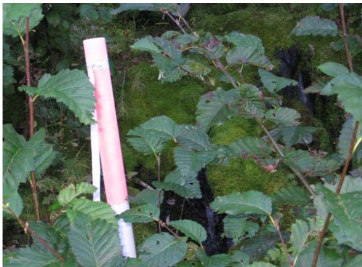
Photo 010 Upstream of inlet – vertical seep.
