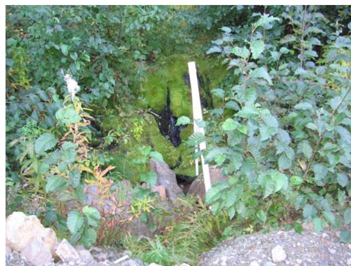
Photo 013 Upstream of inlet – close up of vertical seep.
