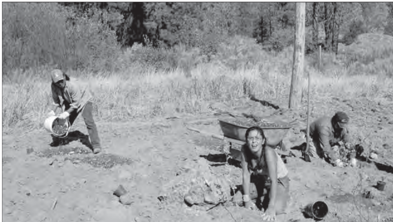
Left to right: Fred James, Jen Calliou, and John Frank of Cayoose plant native seedlings at the powerhouse foreshore restoration site.
