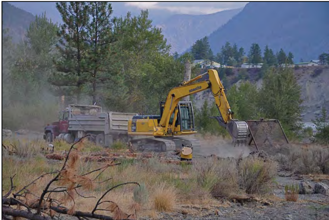
Fig 42 Machine work being carried out on old roadbed, showing native species in foreground
