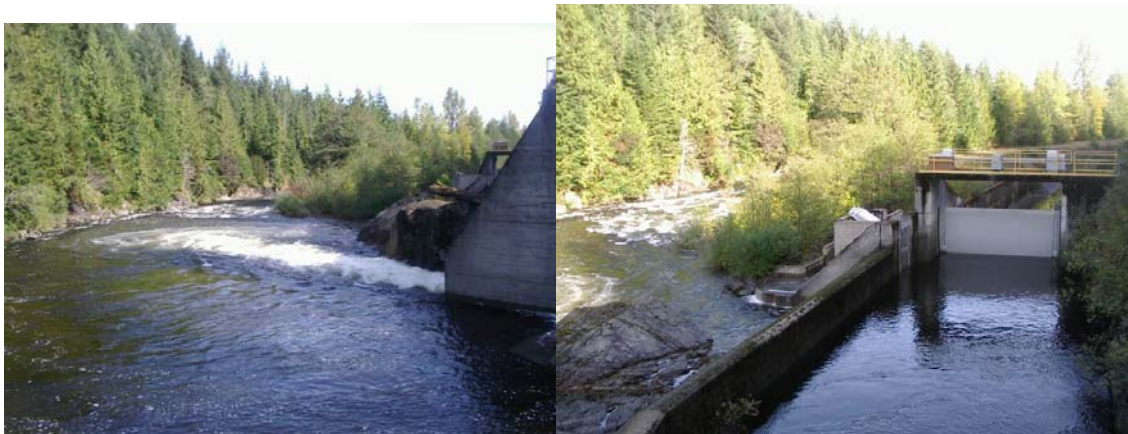
Figure 10. October 8, 2008- undersluice open 0.91m. 16\text{m}^3/\text{sec} all through undersluice and fishway, no diversion flow.
