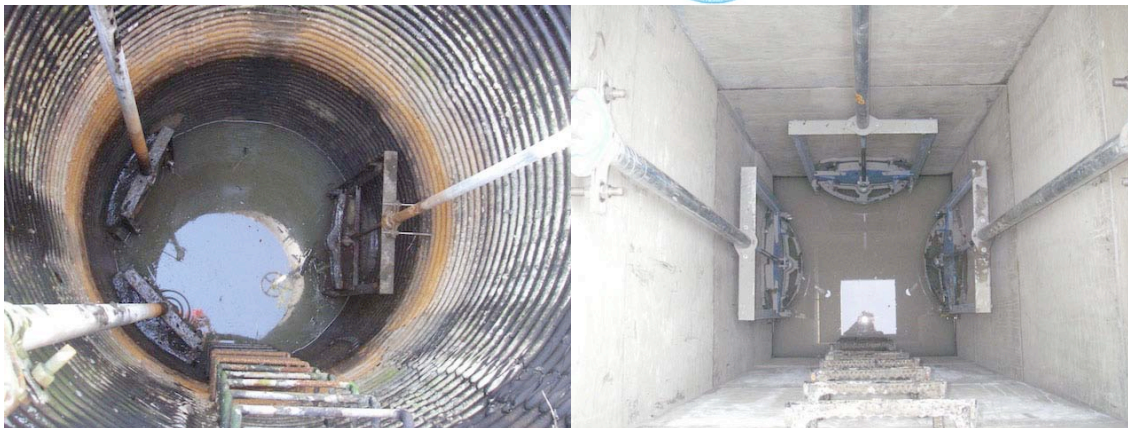
Figure 12 Old galvanized water control with old slide gates and new concrete water control with new slide gates.
