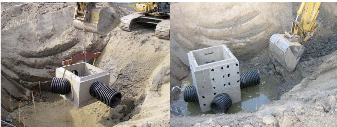
Figure 6 Main concrete control structure being put in the ground (left) and second section added (right).
