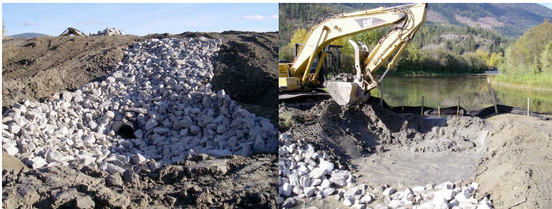
Figure 10 Riprap around the outlet to the Kootenay River (left) and earth dam on Kootenay River side being removed.
