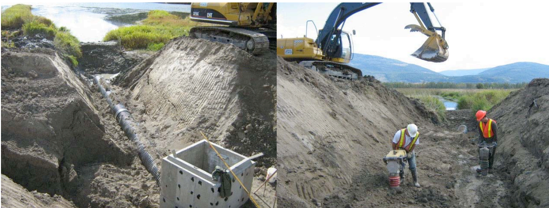
Figure 8 Outlets to pond 3 (left) and pond 4 (right) being put in the ground and buried on 7 and 8 October 2008.
