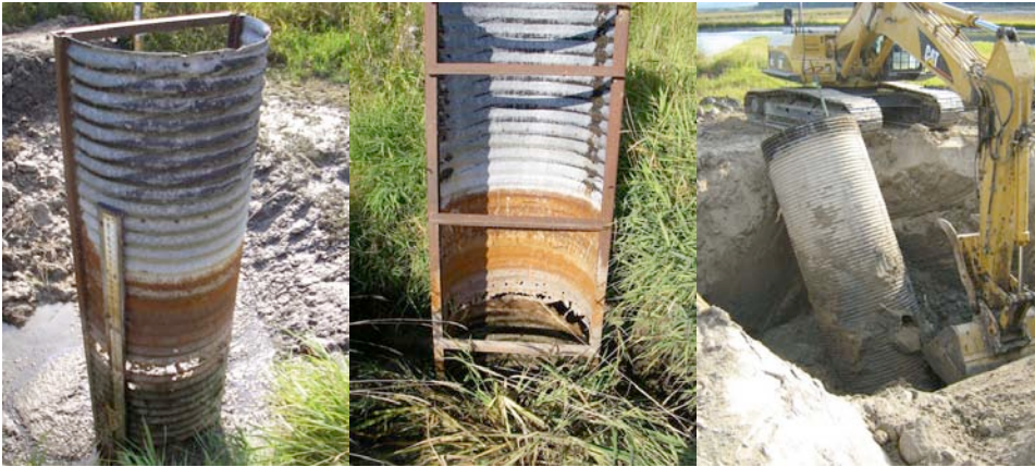
Figure 5 Old perforated half-round stop log structures (left and center) and 3-way control (right) before and during removal.
