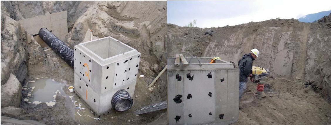
Figure 7 Seepage collar on pipe (top left) and worker compacting the ground with a jumping jack (right).
