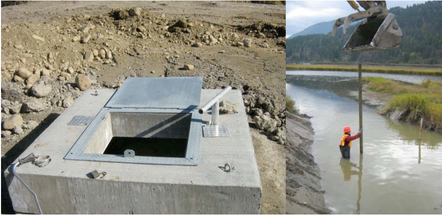
Figure 11 A lockable cover was put on the control structure (left) and a new staff gauge near the outlet to pond 3 was installed (right).
