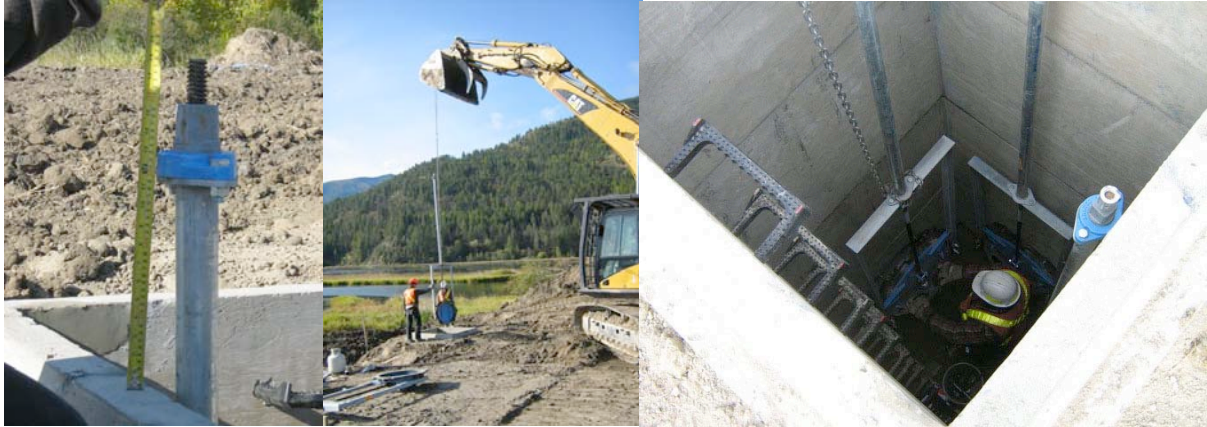
Figure 9 Photos showing the length of stem that was removed (left) on all 3 gates, and slide gate being lowered (center) and anchored to the concrete structure (right).
