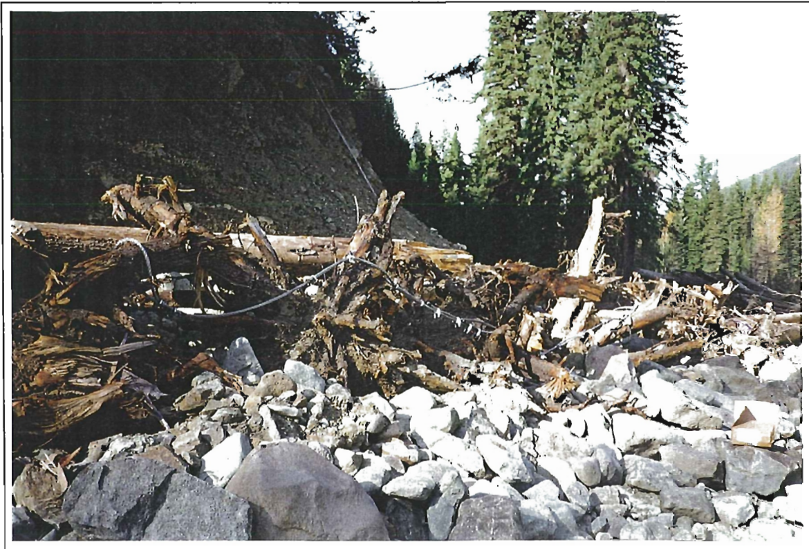
Photo 25: Granite Creek. View of Section 3 facing stabilized west bank. Note: Galvanized steel cable. (20 October 1997).
