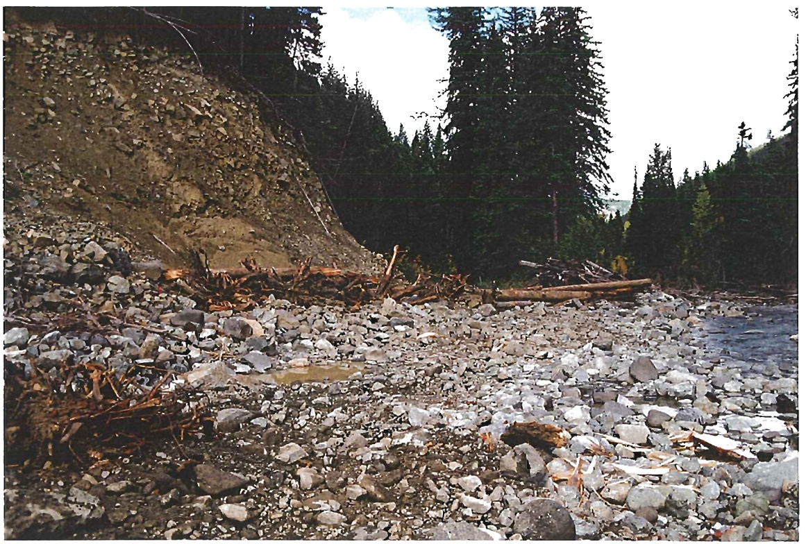
Photo 23: Granite Creek. View Section 3 facing downstream. Post construction. Note: Placed logs extend across dry side channel entrance. (25 September 1997).
