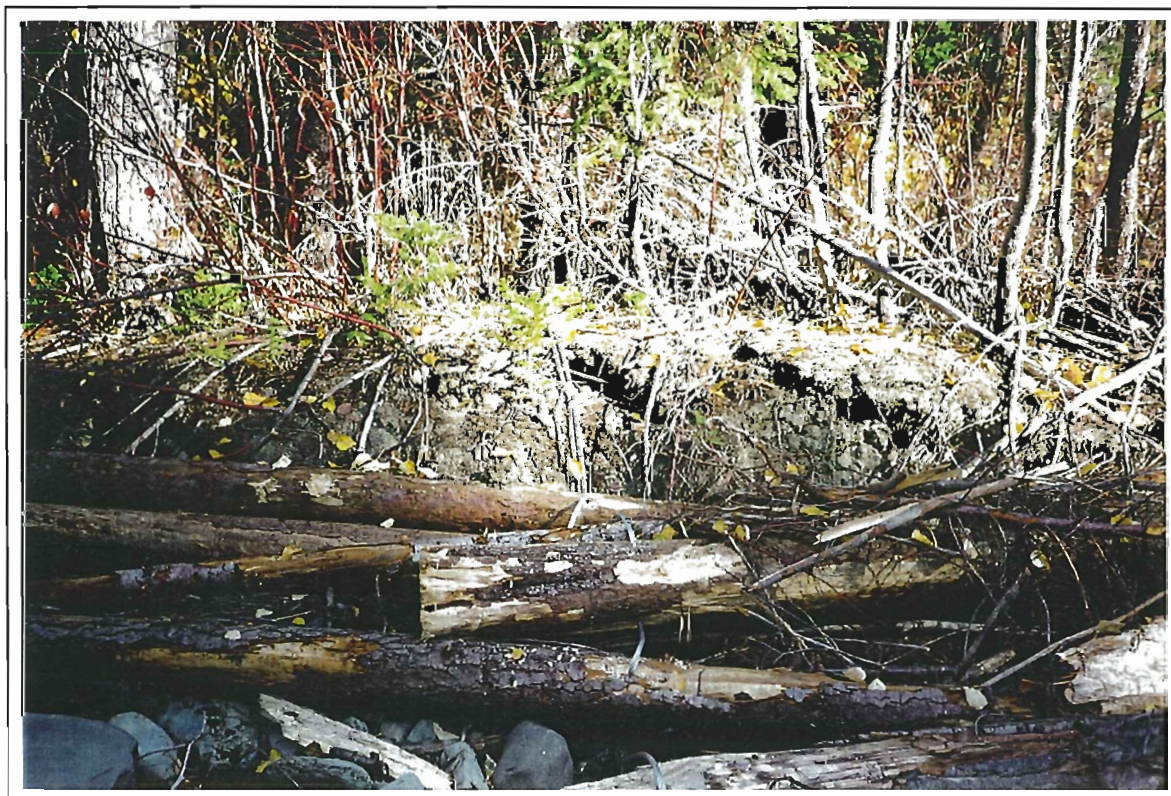
Photo 16: Granite Creek. View of Section 1 facing east bank. Post-construction. Note: Galvanized steel cable. (20 October 1997).
