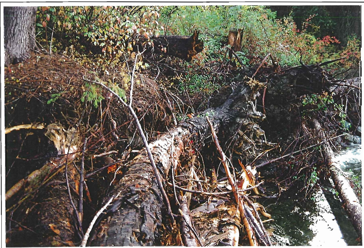
Photo 30: Granite Creek. View of Section 4. Post construction. Note: Logjam has been fortified with logs. (25 September 1997).
