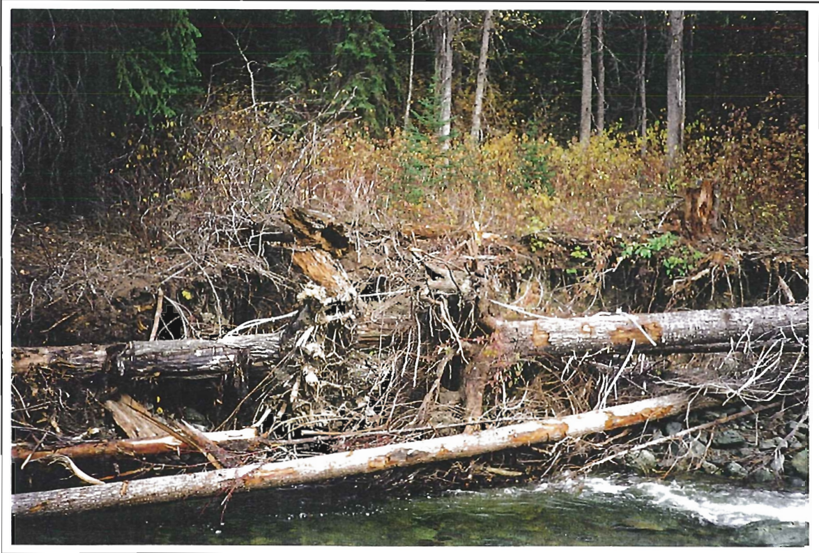
Photo 31: Granite Creek. View of Section 4 facing east bank immediately upstream of logjam. Post construction. Note: Galvanized steel cable. (20 October 1997).
