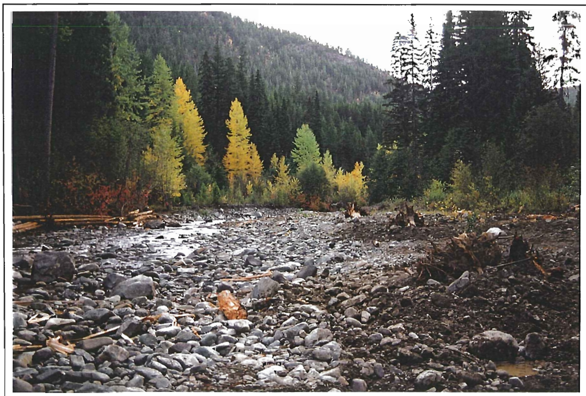
Photo 18: Granite Creek. View of Section 2 facing upstream. Post construction. Note: Rootwads and planted nursetrees. (26 September 1997).
