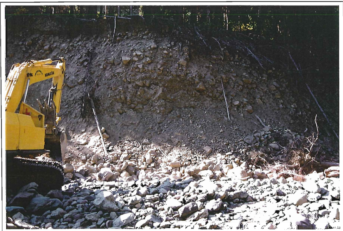
Photo 20: Granite Creek. View of Section 3. Pre-construction. Note: Eroding west bank and excavator. (25 September 1997).
