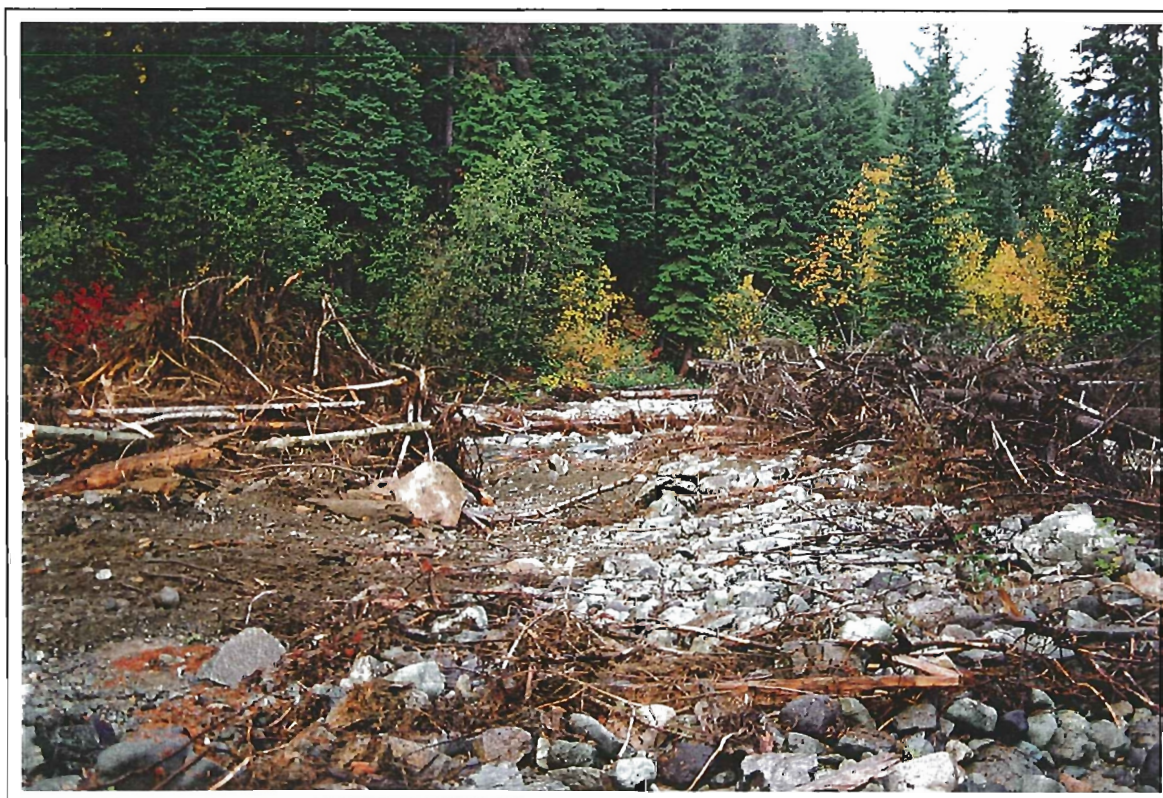
Photo 38: Granite Creek. View of Section 6 facing downstream. Post construction. Note: East bank stabilized with logs and debris. (26 September 1997).
