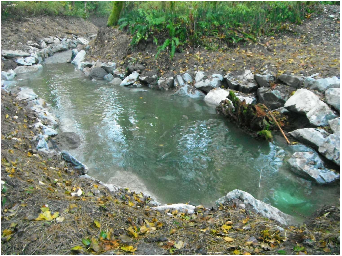
Intake pipe (facing downstream along newly constructed intake channel – note armour and spawning riffle further downstream)
