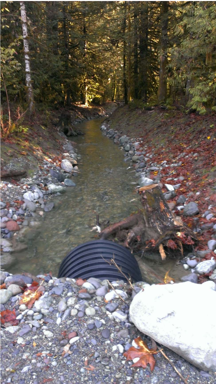
Newly installed PVC Culvert at northern end of project site (on SD#44 school property)
