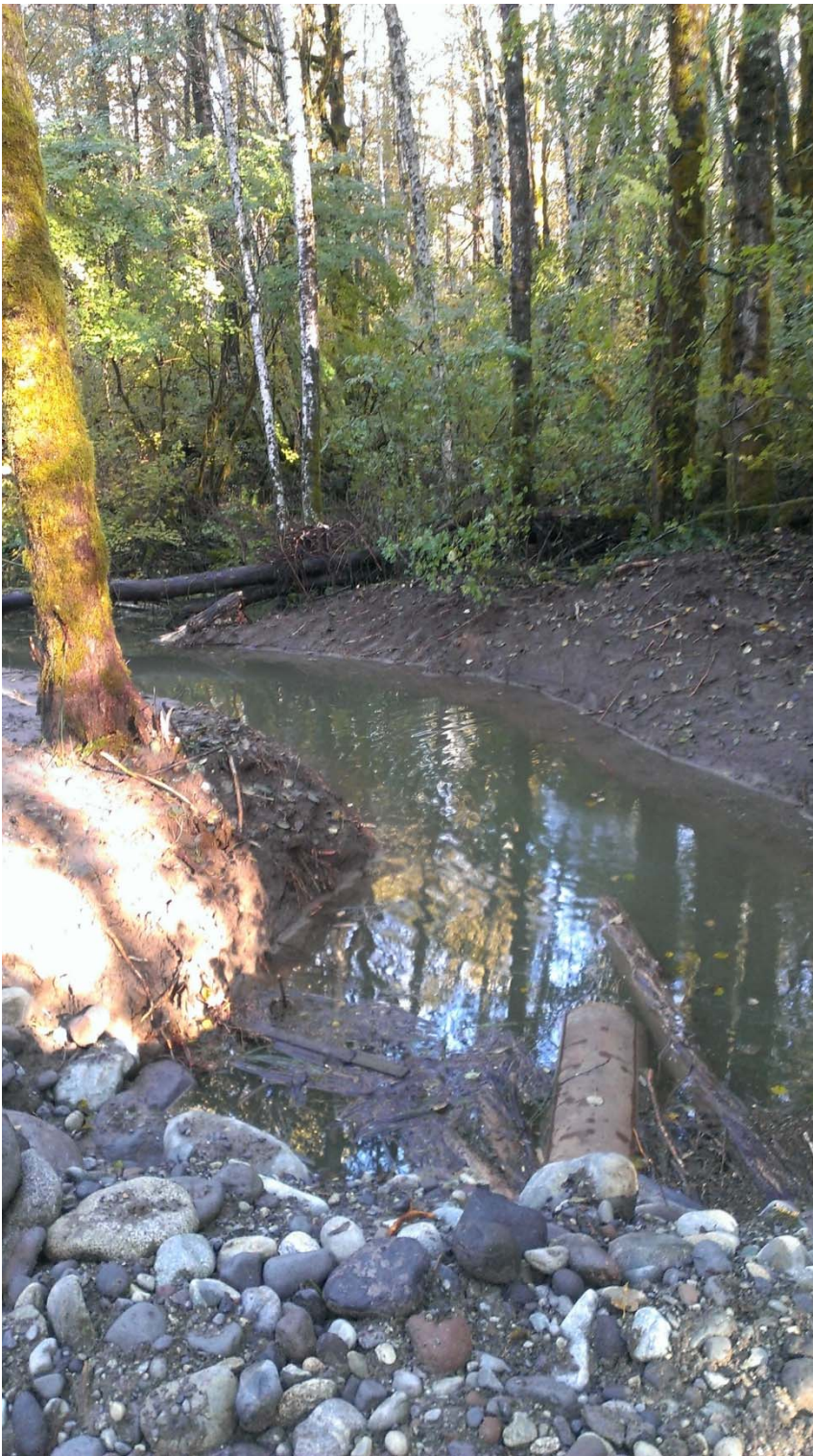
Facing upstream from road/train/top of dike; note newly installed steel pipe intake
