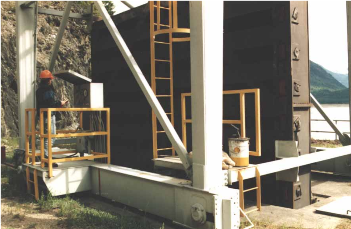
Plate 10. The Low Level Operating Gate (LLMG) being lowered to begin a fish transfer.
