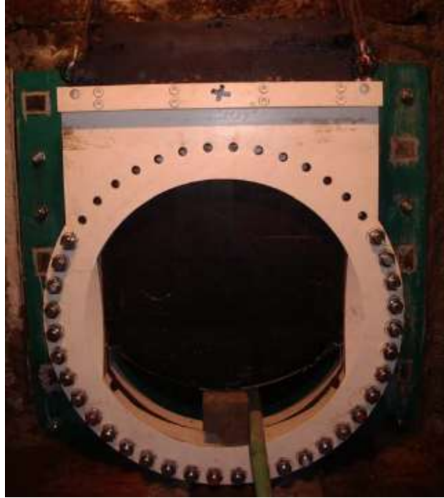
Figure 7 Knife gate valve installed in 2008 at one of the LLOs in the Coquitlam Dam gatehouse (BC Hydro Engineering 2009).
