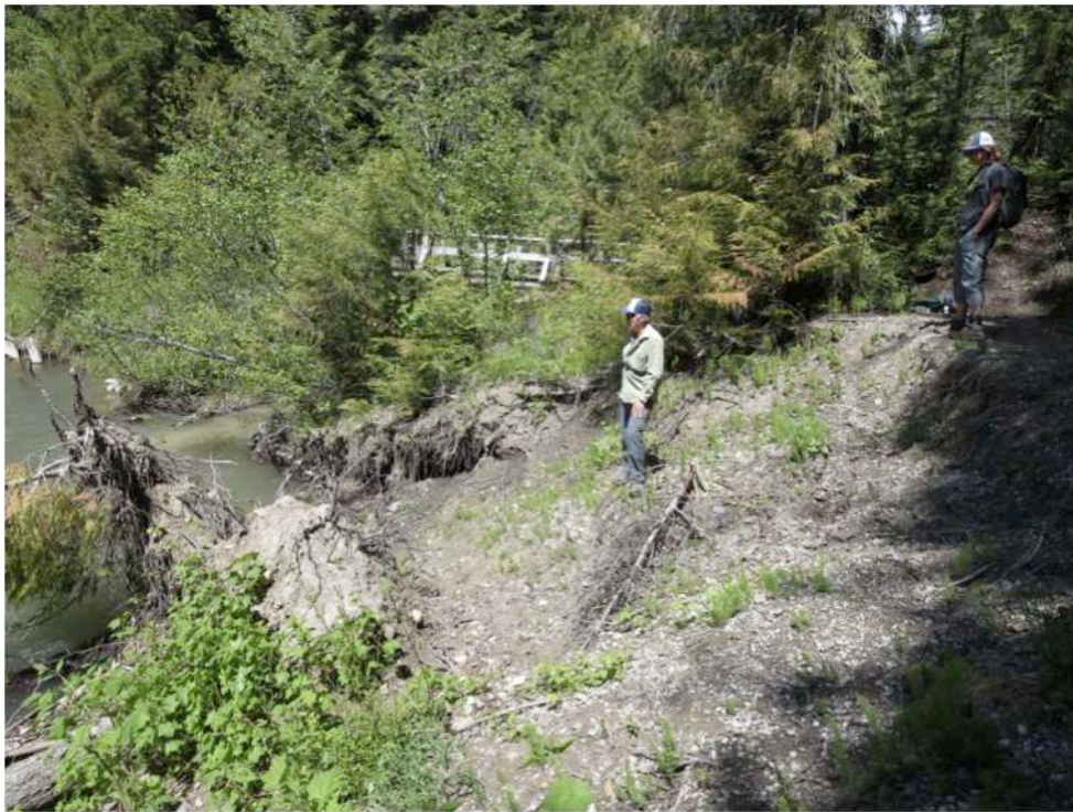
Figure 6 - Photo of Site 2 Slope Failure, July 2014
