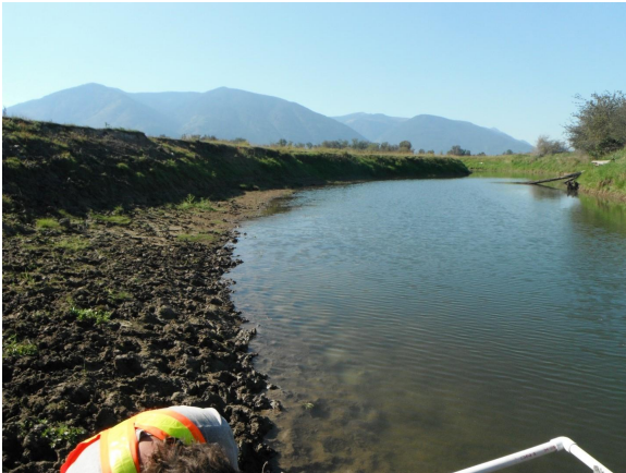
Photo 12. Close up view of oversteepened banks and exposed soils.
