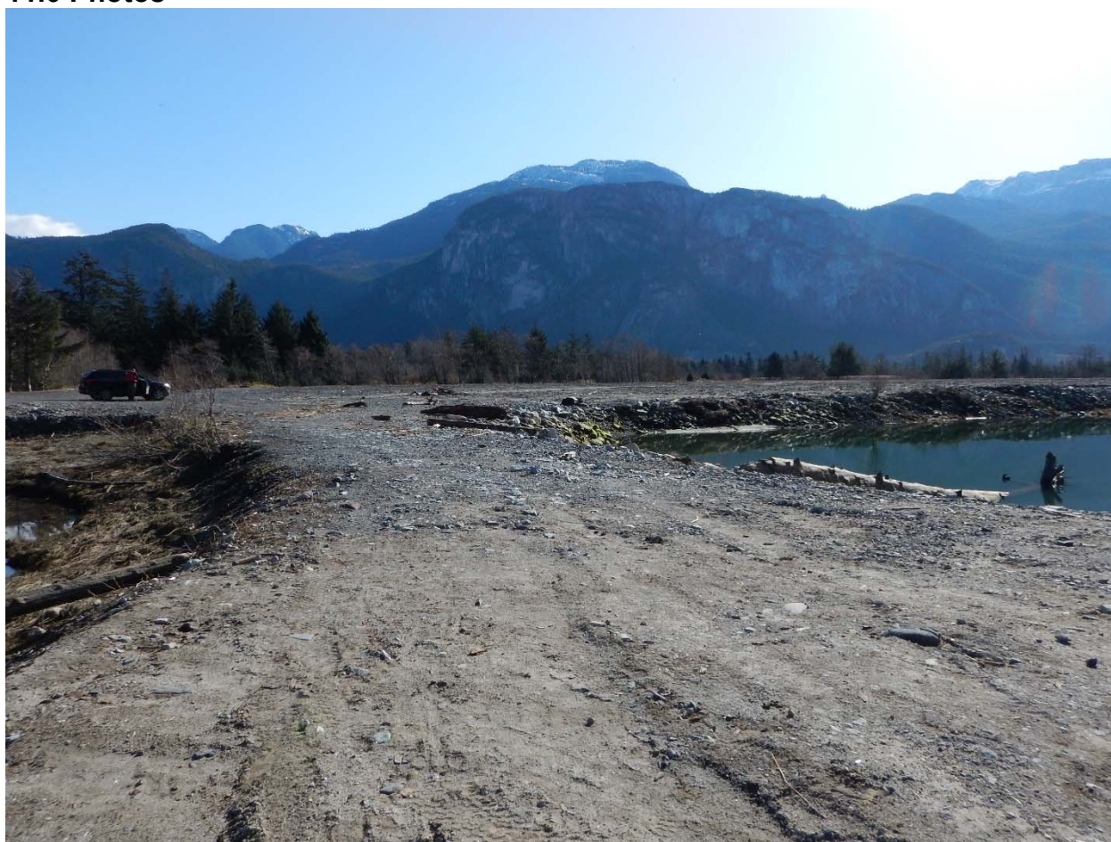
Photo 12. March 2, 2015 – prior to construction. Facing east from berm at north end of log-dump pond
