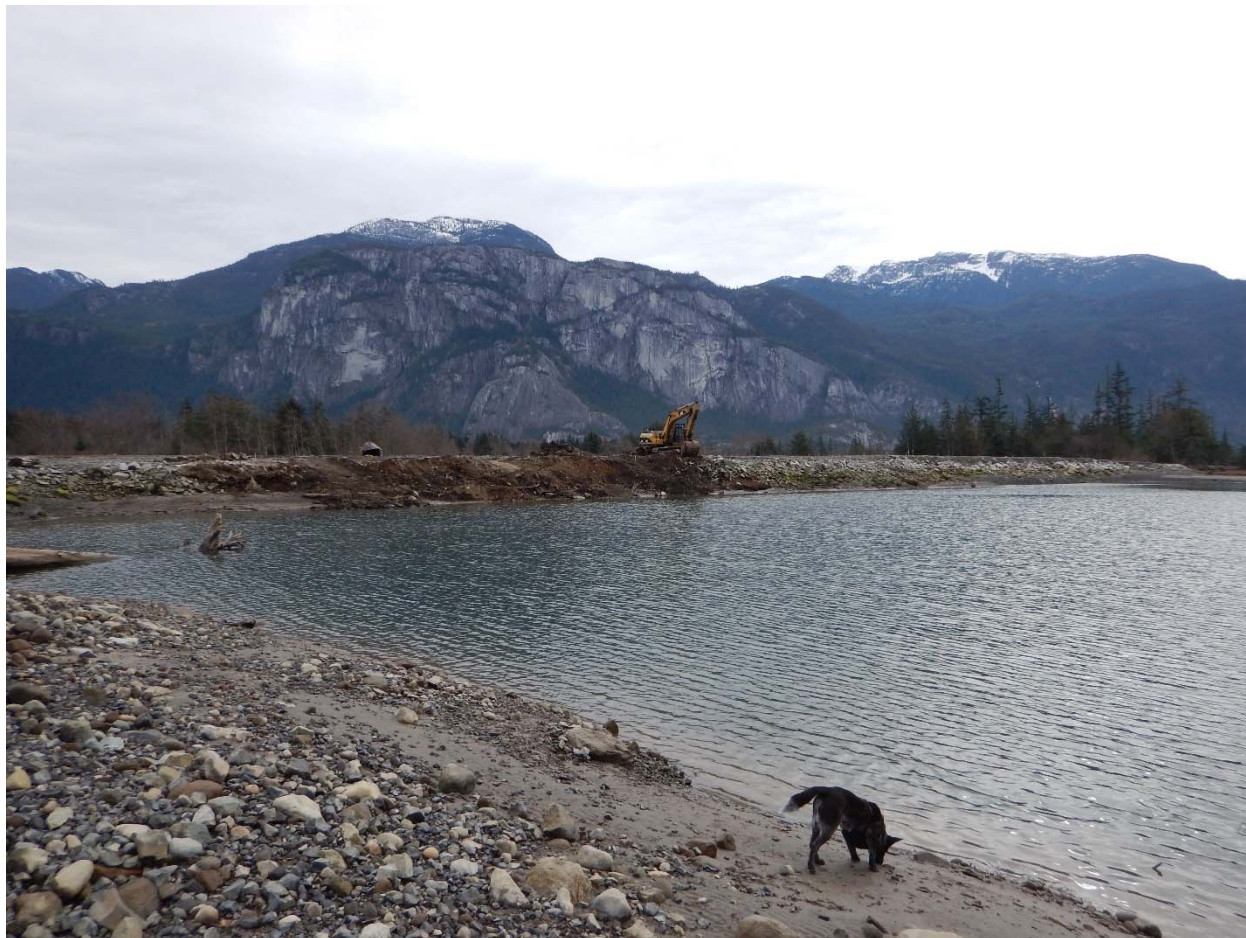
Photo 13. March 5, 2015 – Construction just starting. Facing east from berm north of log-dump pond
